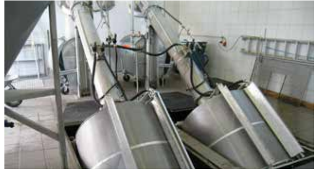
Low space requirement due to the use of two HUBER Rotary Drum Fine Screen ROTAMAT in the channel, size 1400.
