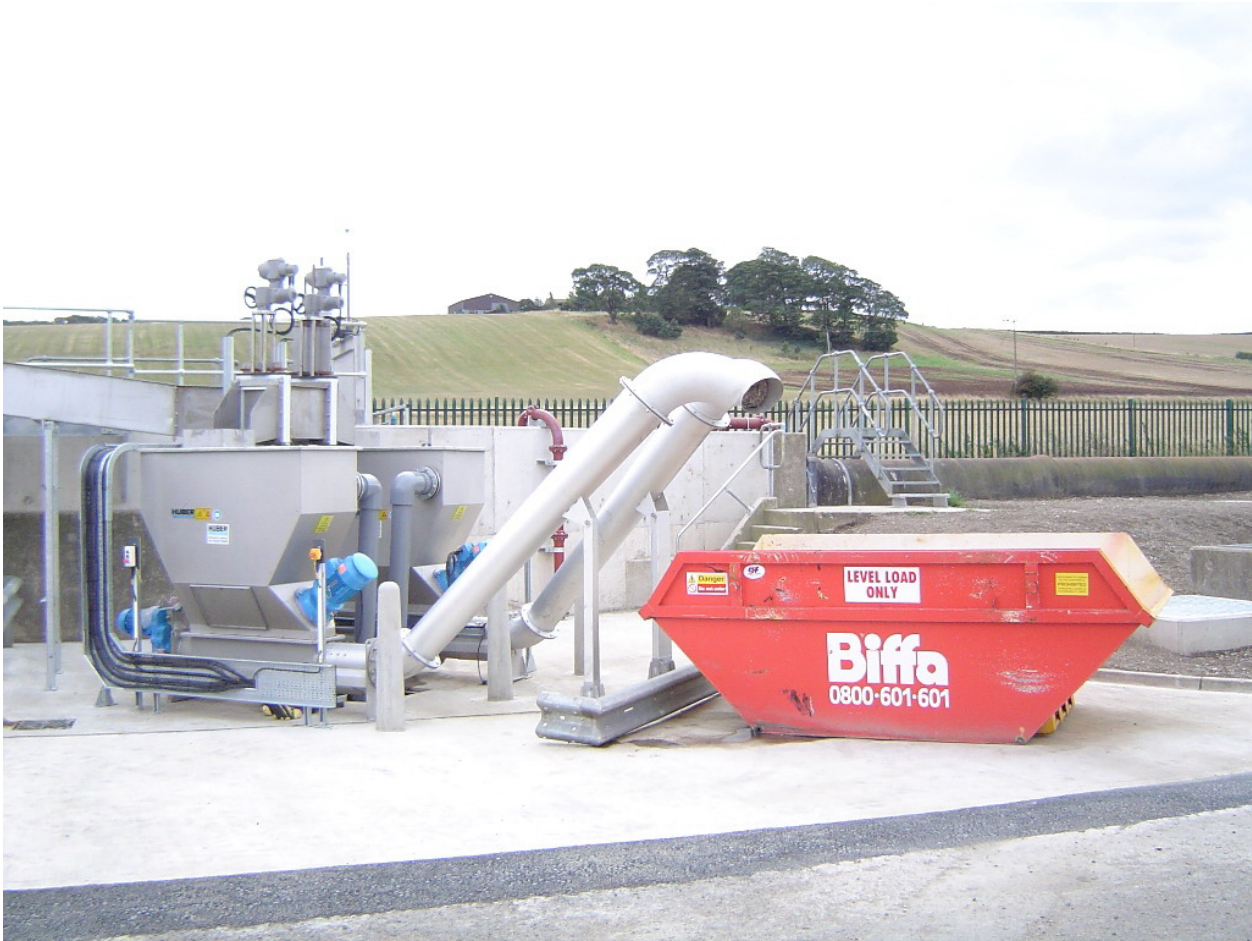
Fig. 2: Super-laundry wash-presses fed through a sluice channel (Huber Technology)
