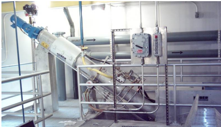
Figure 36 – Rotary Perforated Plate Screen at Belle Plaine, MN
