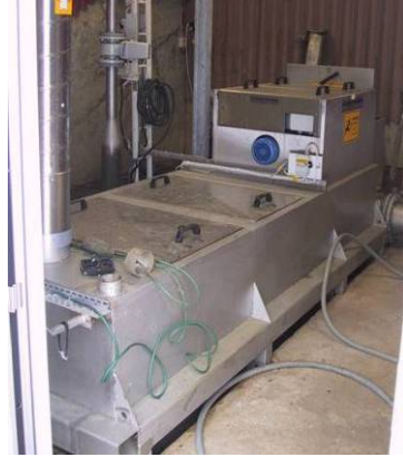
Figure 15 – Tank mounted Step screens
