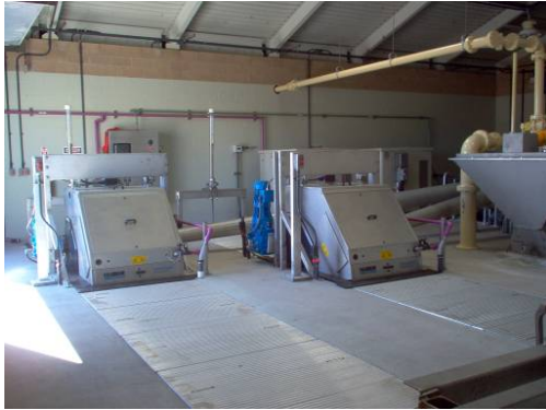
Figure 6- Step Screen at Reno Stead, NV
