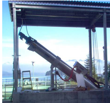
Figure 4- Ro2 installation in Alaska (with frost protection package)
