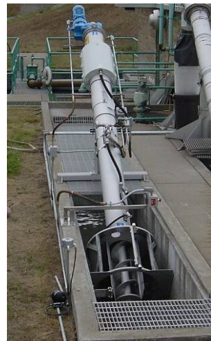
Figure 2: Huber ROTAMAT® Fine Screen Ro1 installed at Merrill, WI
