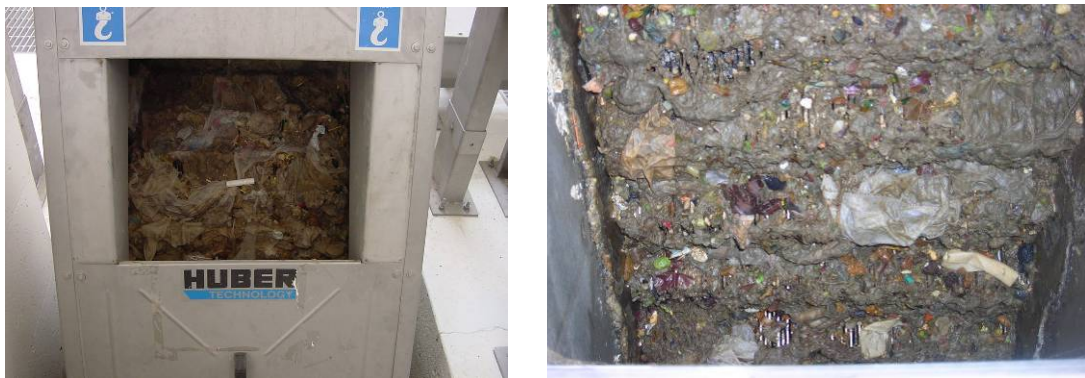
Figure 12, 13 – Proper screenings mat for a Step Screen
