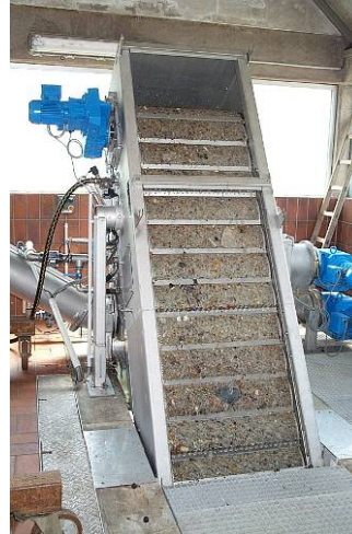
Figure 21 – Perforated band screen (covers removed)
