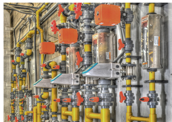
Millennium III ClO 2 Generators provide pre-oxidation and disinfection at the Otay Water Treatment Plant
