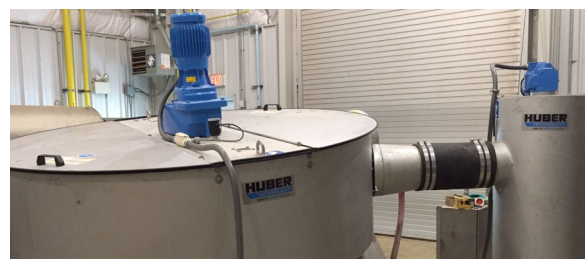
Wildcat Hill Water Reclamation Plant Location: Flagstaff, Arizona
