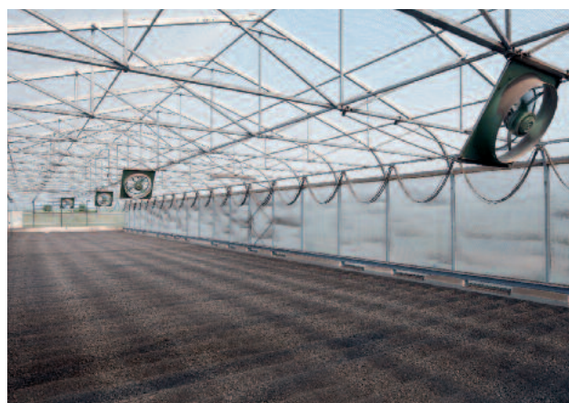
Ventilators blow dry air over the sludge bed.
