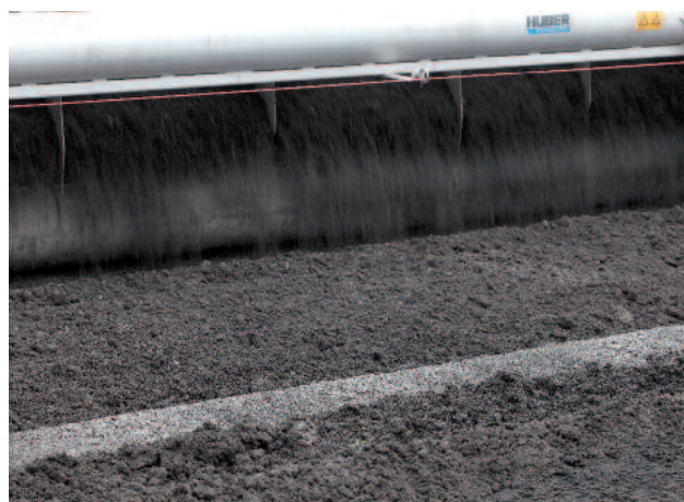
Backmixing and aeration of sludge
