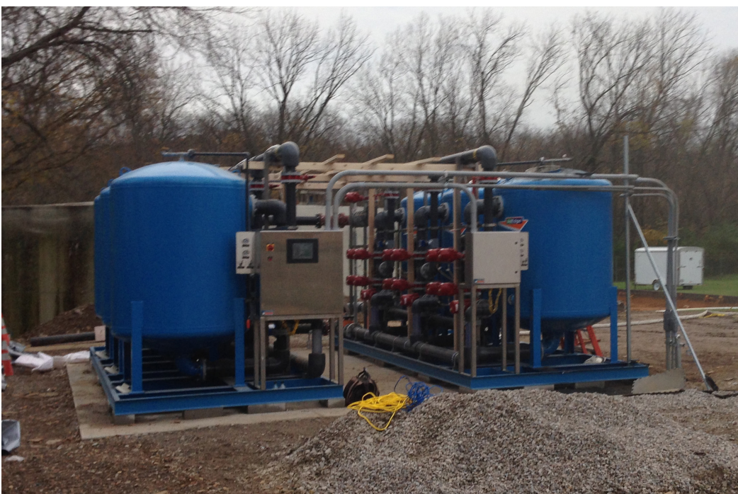
AdEdge Water Technologies, LLC provided two triplex systems for the Aqua OH - Worthington Hills community.
