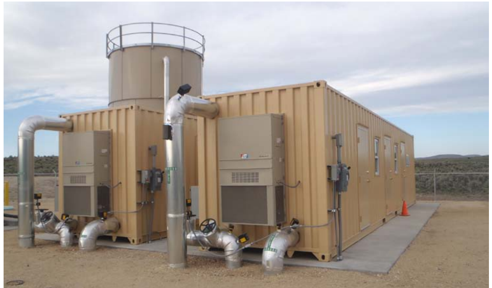
Each WaterPOD contains an AdEdge GS+ coagulation/filtration package sized for the well's maximum combined flow of 1,950 gpm.
