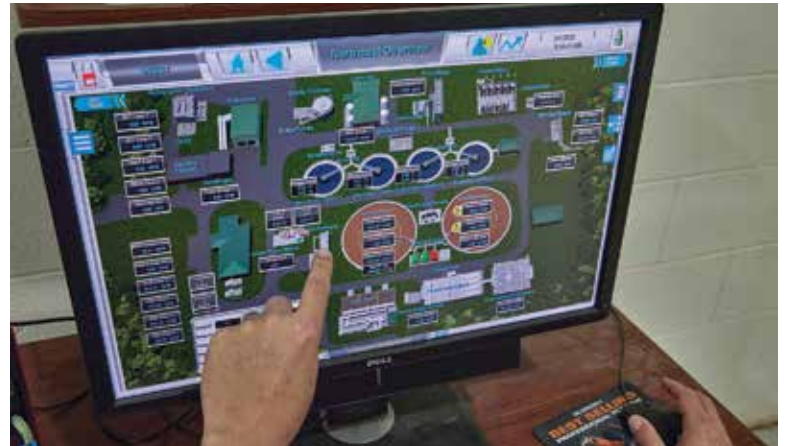
The plant has multiple monitoring stations. It is operated and manned around the clock. (SCADA display supplied by MR Systems)
