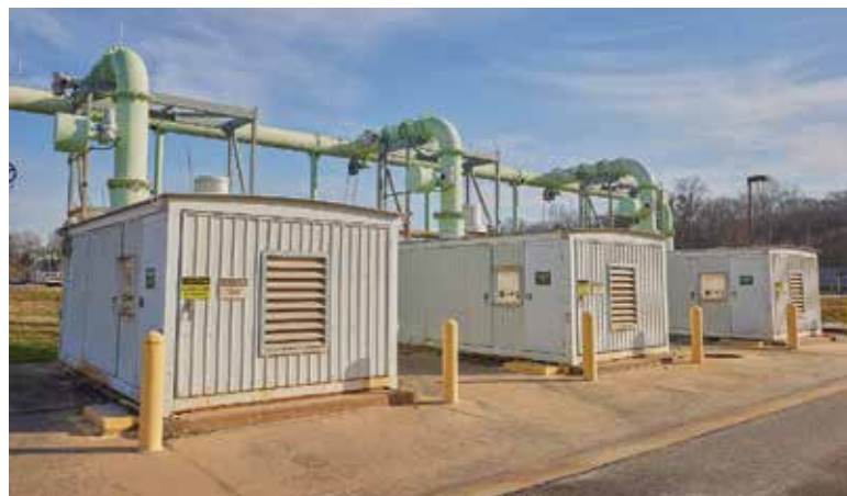
Turblex/Howden Roots aeration blowers provide aeration for the secondary treatment process.
