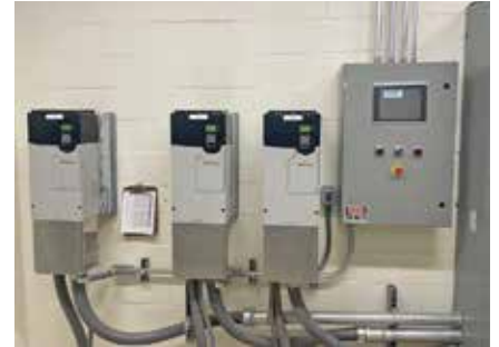
The stacked units are plumbed to operate individually or collectively. The facility team was able to plumb into the existing air manifold.
