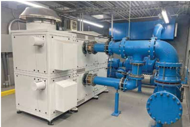
The facility team left one of the existing multi-stage blowers positioned next to the new Inovair units for extreme backup purposes.
