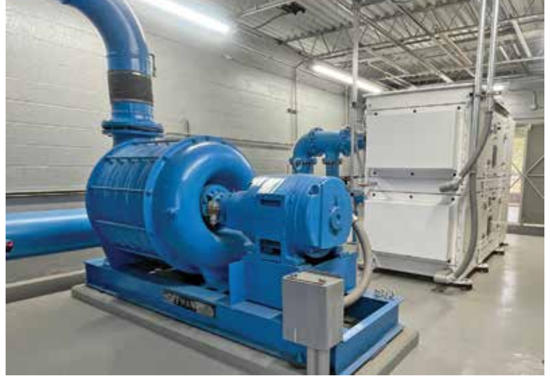
The stacked blowers (Inovair) in place and operational.
