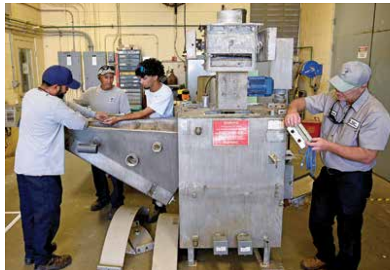
Jonathan Perez, Pablo Pagan, Lucas Perez and Richard Craig perform maintenance on a slaker at the Corkscrew plant.
