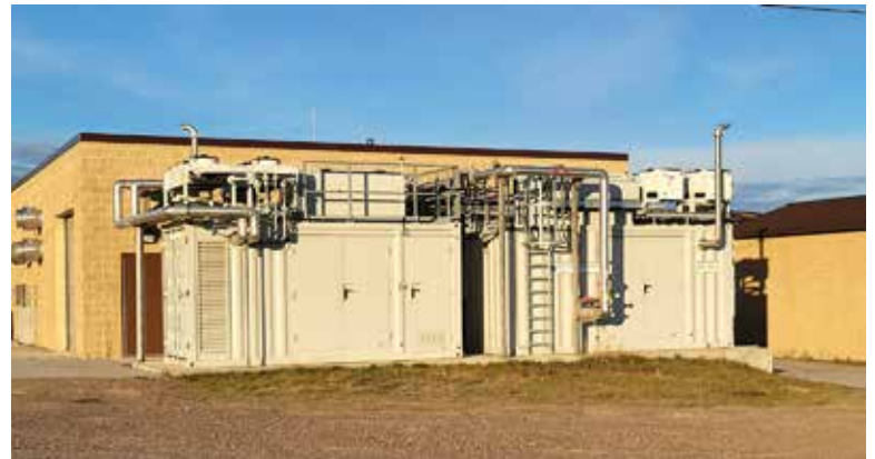
The two 100 kW generators at the food waste processing building at the Kinross Wastewater Treatment Plant produce heat and power.
