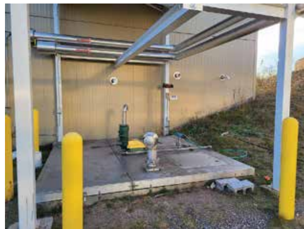
A FOG receiving station was recently added to the site.
