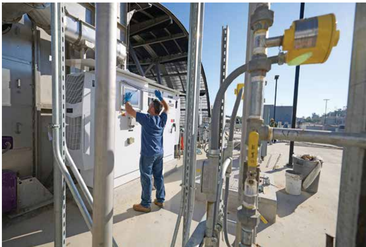
Jason Haddix, operations supervisor, near the secondary sedimentation tanks at the wastewater treatment facility. (Brackett Green Drum Screen from Ovivo.)
