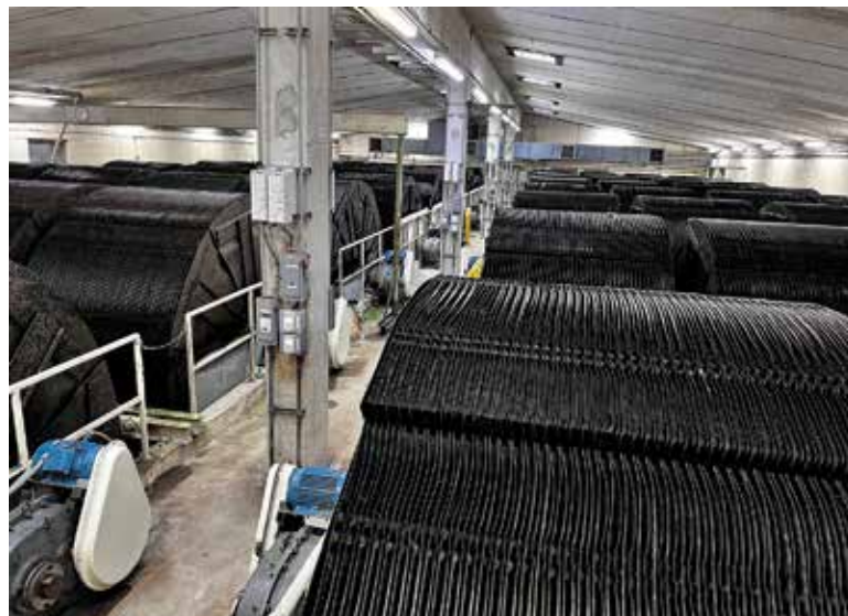
Rotating biological contactors provide secondary treatment at the Penn Yan facility.
