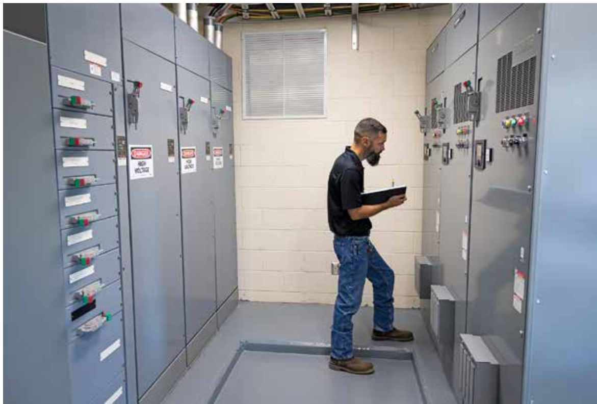
Jared Duncan, one of 39 South Walton Utility team members, records electrical data on the pumps and motors at the Goldsby Road pumping station.
