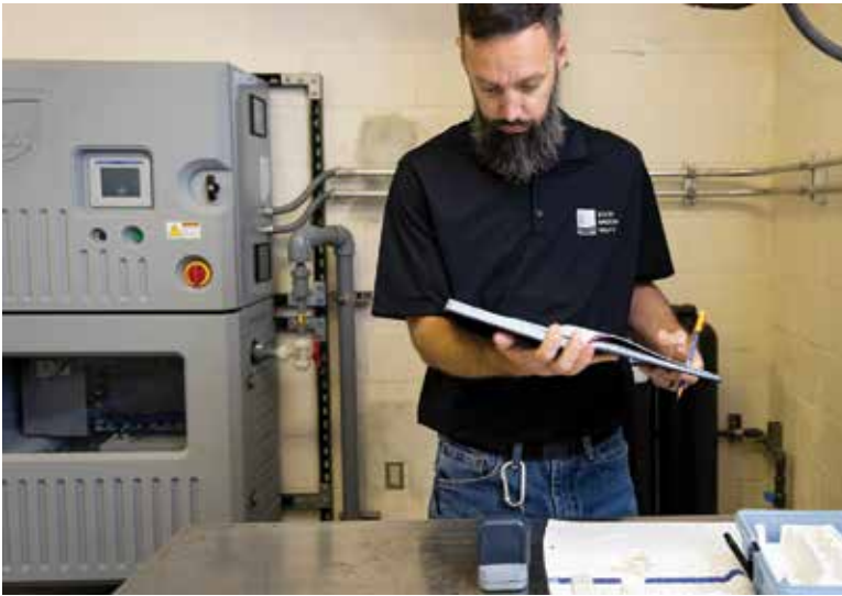
Duncan checks the chlorine levels (Regal injection system from Chlorinators Incorporated) at the Goldsby Road pumping station. (MIOX water chlorination generator from De Nora)
