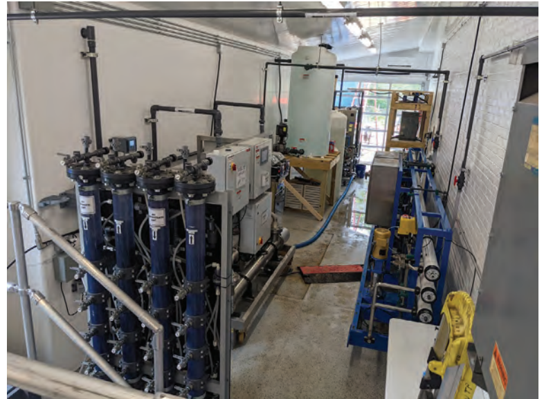
The PUREWater Westminster pilot project is a 20 gpm version of what the city hopes will become Maryland's first indirect potable reuse project. The goal is to supplement the city's water supply with up to 1 mgd.
