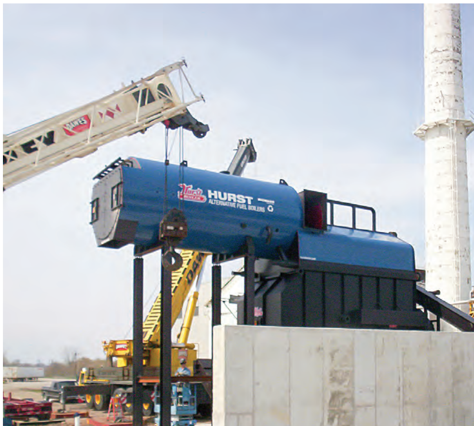
A Hurst Boiler & Welding Co. Inc. 1,500 hp boiler is delivered to ST Paper, Oconto Falls, Wisconsin.
