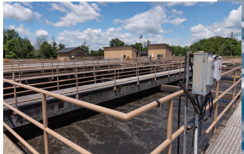
The Allenstown plant has a design capacity of 1.5 mgd and an average flow of 0.62 mgd.
