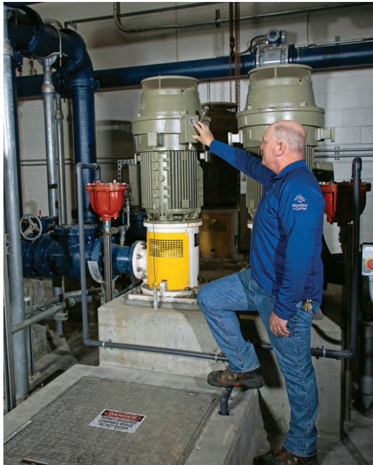
Sullivan checks the lubricant level in one of the three finished water pumps (Sulzer Pumps Solutions) in the plant’s process area.
