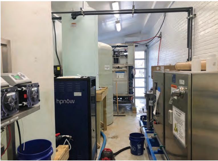
Another view of equipment in Westminster’s pilot project for indirect potable reuse.
