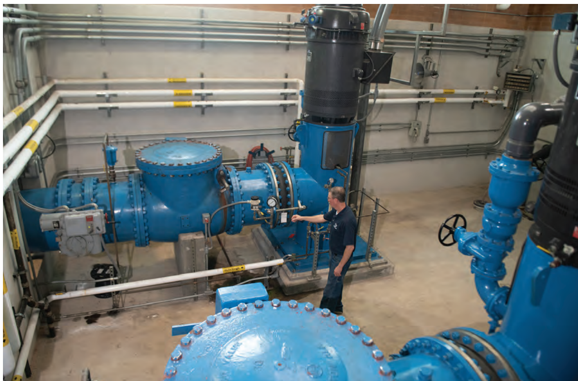
The Marston plant's backwash water supply system uses a Peerless pump driven by a motor from US Motors (Nidec).
