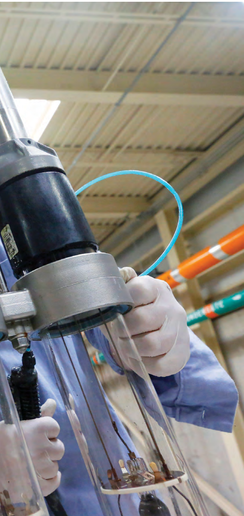
Brad Daroci, with the maintenance department, cleans the UV lamp system (TrojanUV4000Plus) in the UV building at the Downriver Wastewater Treatment Facility.
