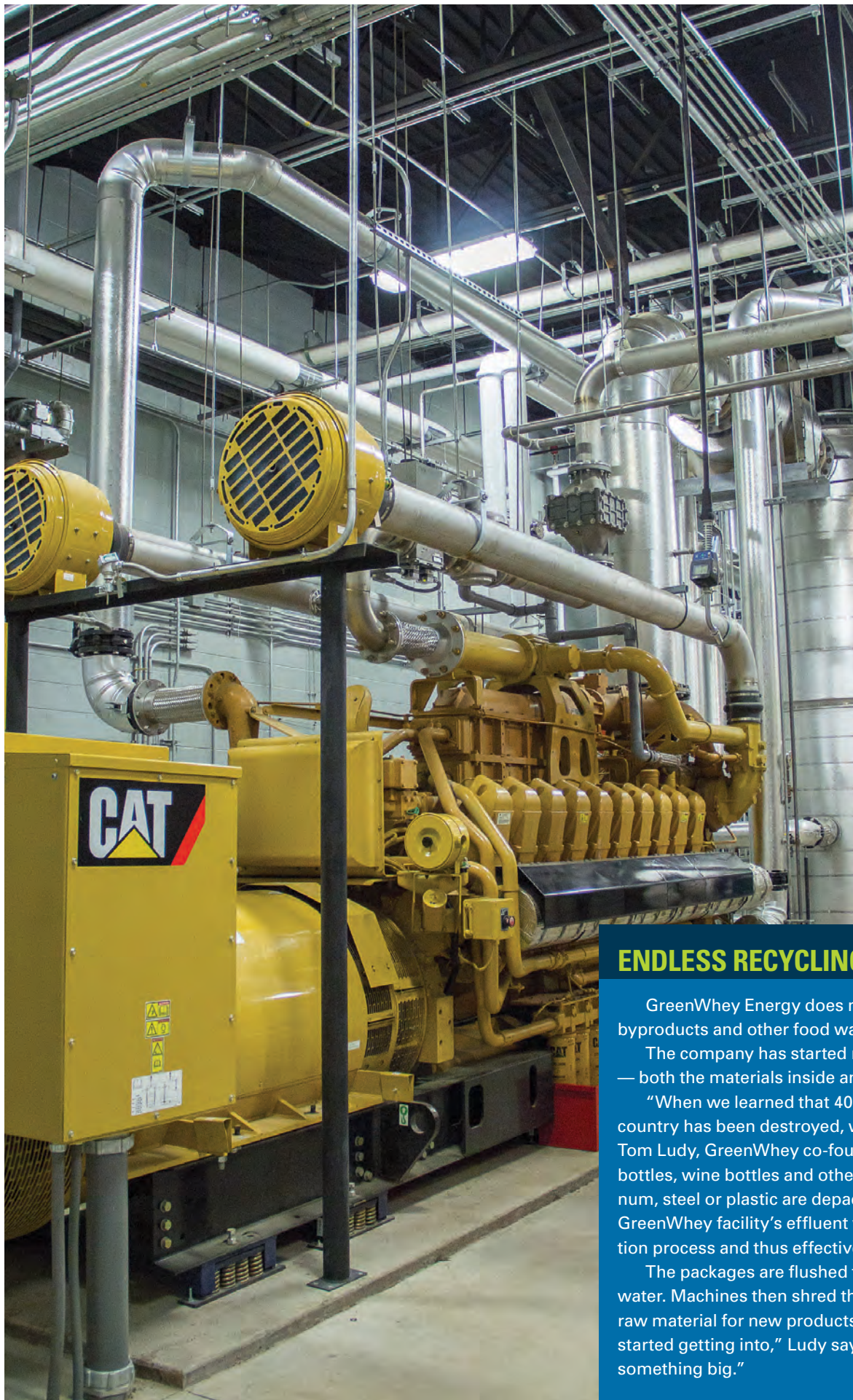
Two Caterpillar biogas-fueled generator sets like this one produce electricity at GreenWhey.
