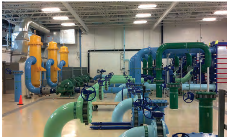
The Centralized Renewable Energy System on the Innovation Campus will eventually provide heating and cooling for 1.8 million square feet of building space.
