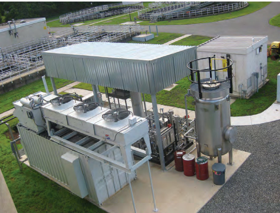
Technology used to convert methane gas to electricity includes anaerobic digesters, a 240 kW engine/generator from Kraft Power, and a 50 kW solar field from Advanced Solar.
