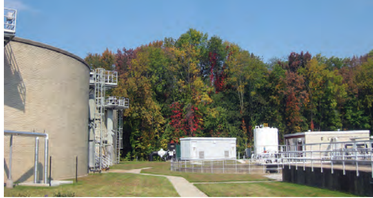
Electricity production is enhanced when food wastes such as fats, oils and grease are added to the process by way of this liquid waste receiving station.
