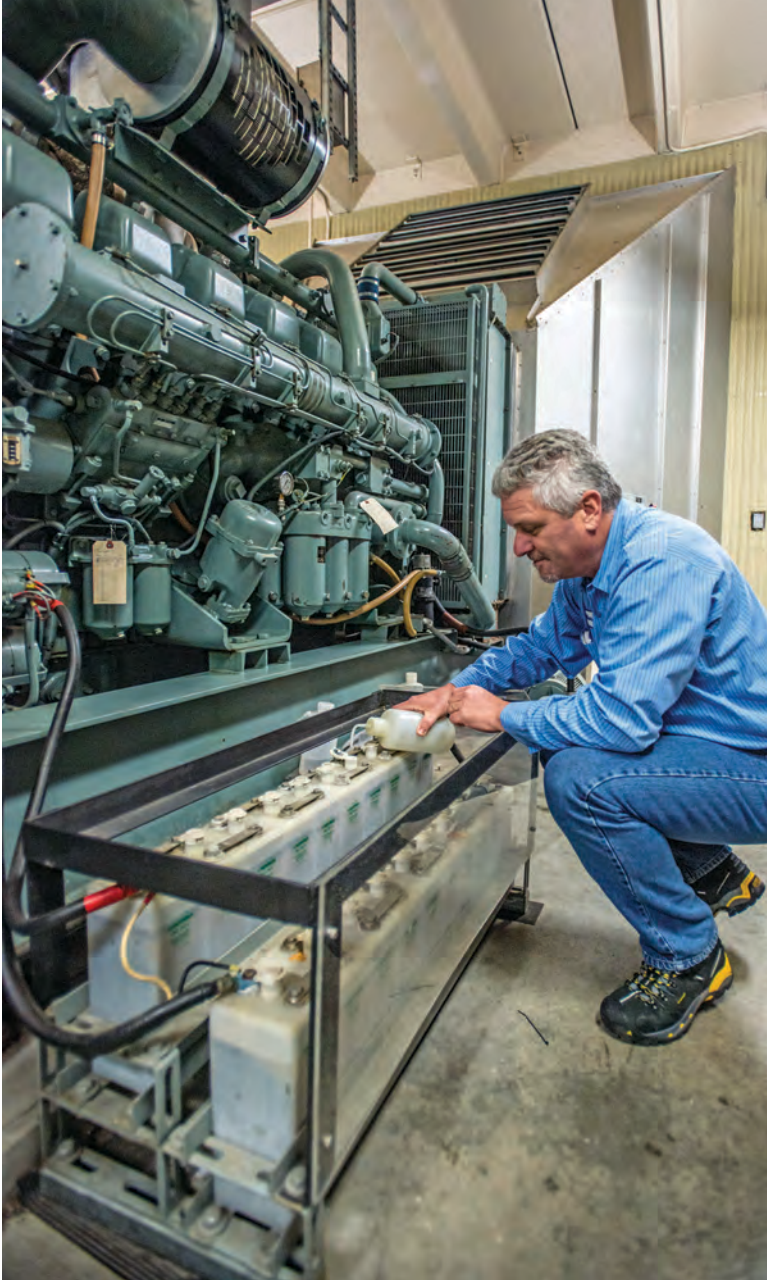
Mark Fogle checks on the plant's emergency generators.
