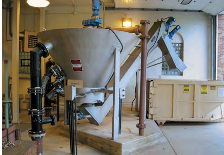
One of two RoSF 4 COANDA grit washer units (Huber Technology). One unit operates at all times. By rotating the units, the plant can keep one on hand for standby and perform maintenance on one unit while the other is online.
