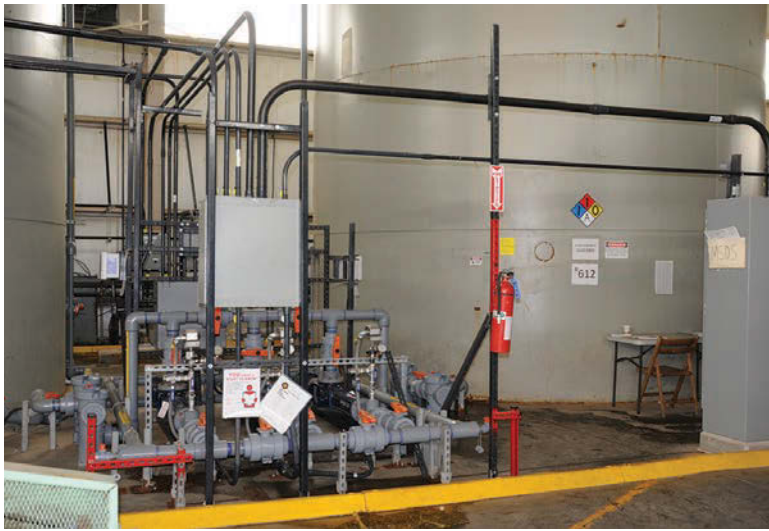
The glycerol storage and piping system.
