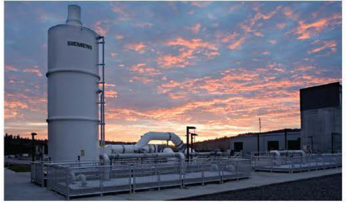
The Siemens odor control system helps the expanded Tri-City Water Pollution Control Plant fit in with the neighborhood, including a $100 million condominium development next door.
