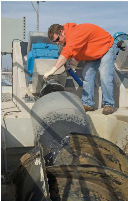
Operator Dan Reinhardt greases screw pumps (Spaans Babcock).
