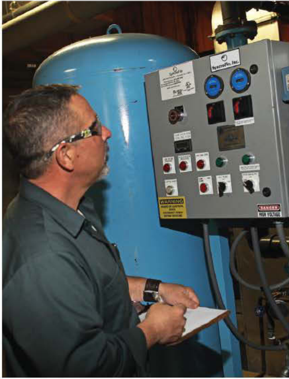
Plant manager Chris Rowe checks the water pump system (SyncroFlo).
