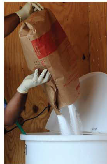
Soda ash from General Chemical Performance Products is added to raise the pH as part of the plant’s approach to reducing zinc in the effluent.
