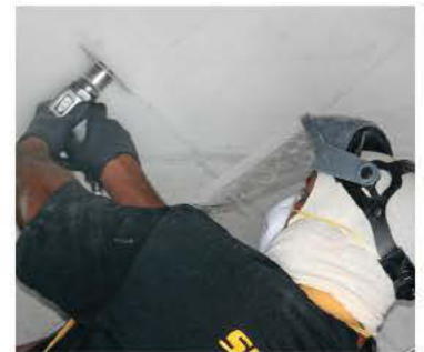
A Conco Spray Solutions crew member cuts grooves into the cleaned and prepped surface before applying the polyurethane coating material to ensure optimum adhesion and uniform coverage.
