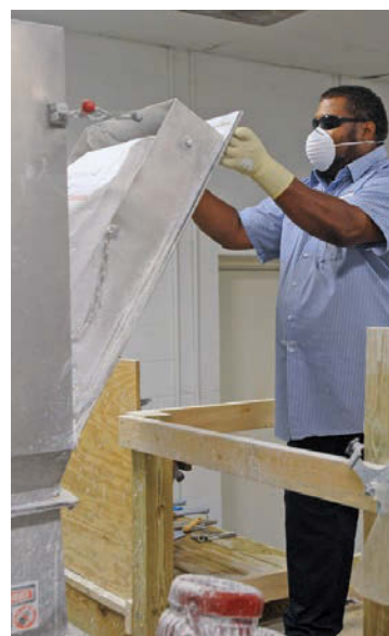
Jerome Houston loads the lime feeder. Lime addition is part of the zinc removal system.
