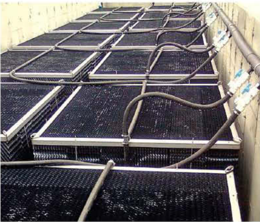
Ball valves in the aeration header (right) control the flow through the feeder lines to the air racks.
