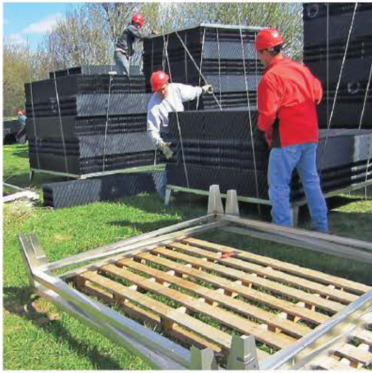
Workers from Penro Construction unload 6-foot-square, 8-foot-tall polishing modules and place them on pallets.
