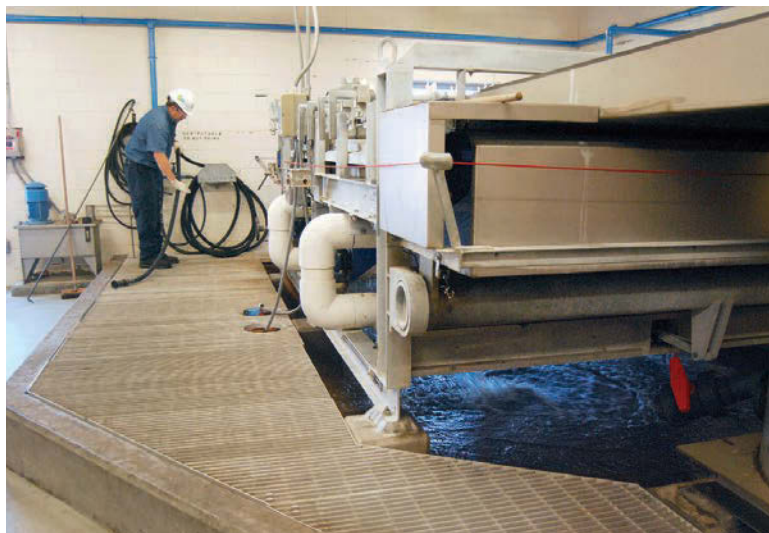
Mark Byrns hoses down the Ashbrook belt press.
