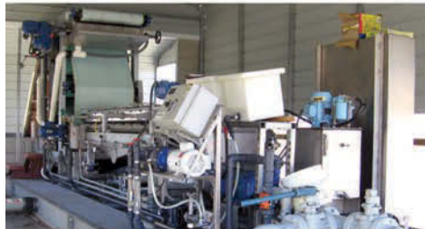
Skid Mounted System Thunder Bay Casino Sacramento, CA Tel: 209-483-4118
