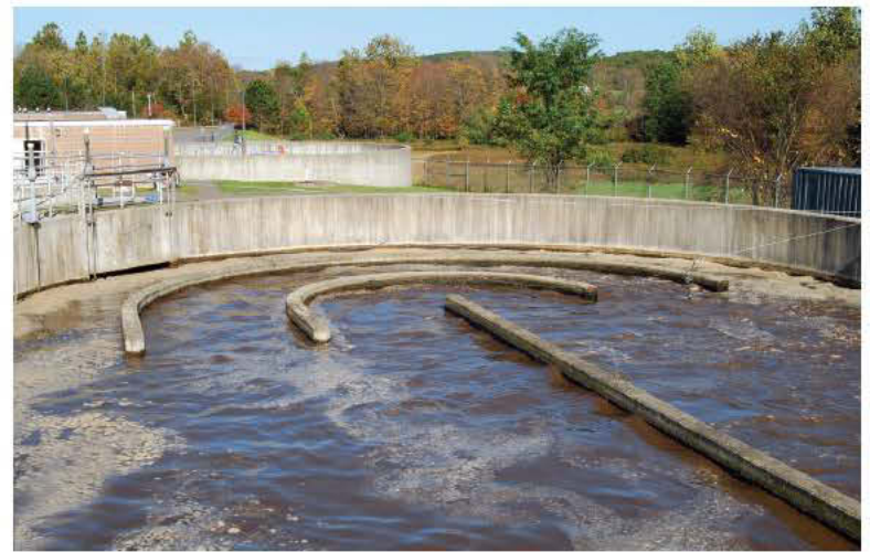
An Ovivo oxidation ditch at the Newtown Wastewater Treatment Plant. The facility, operated by United Water, won a 2009 U.S. EPA regional wastewater treatment plant excellence award.
