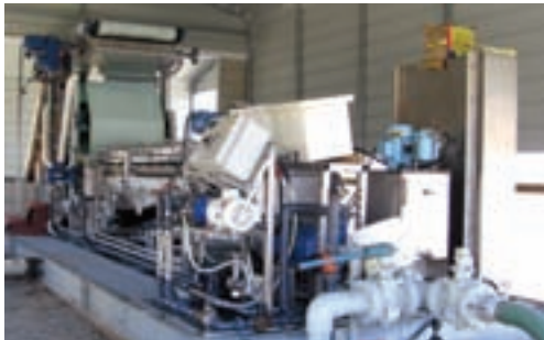
Skid Mounted System Thunder Bay Casino Sacramento, CA Tel: 209-483-4118
