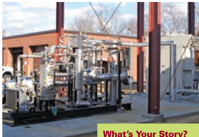
PHOTOS COURTESY OF WILLINGBORO POLLUTION CONTROL FACILITY
