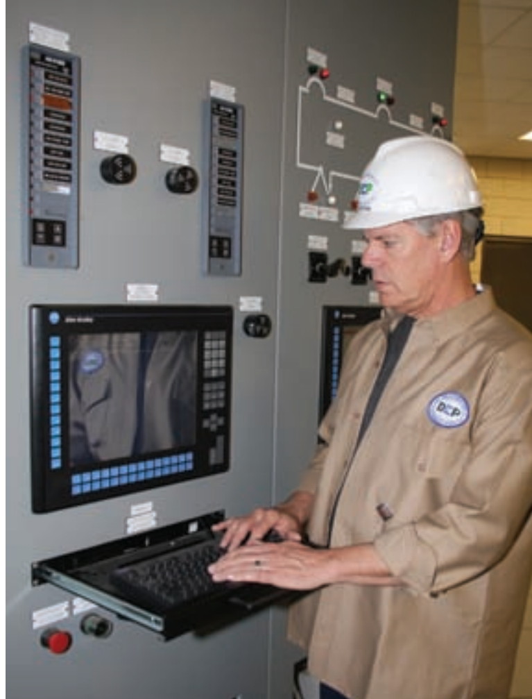
Superintendent Jim Pynn inputs information on the Allen-Bradley control system (Rockwell Automation) in the plant control room.
