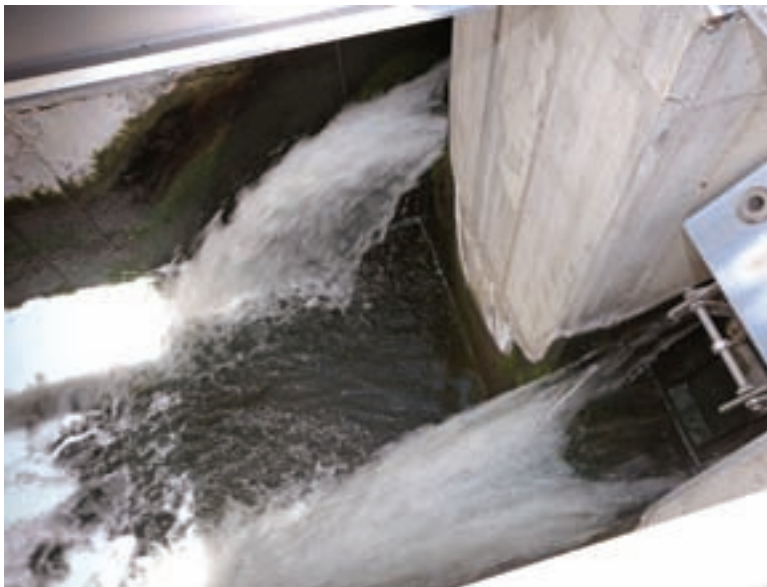
Final effluent after UV treatment and before discharge to the Missouri River.
