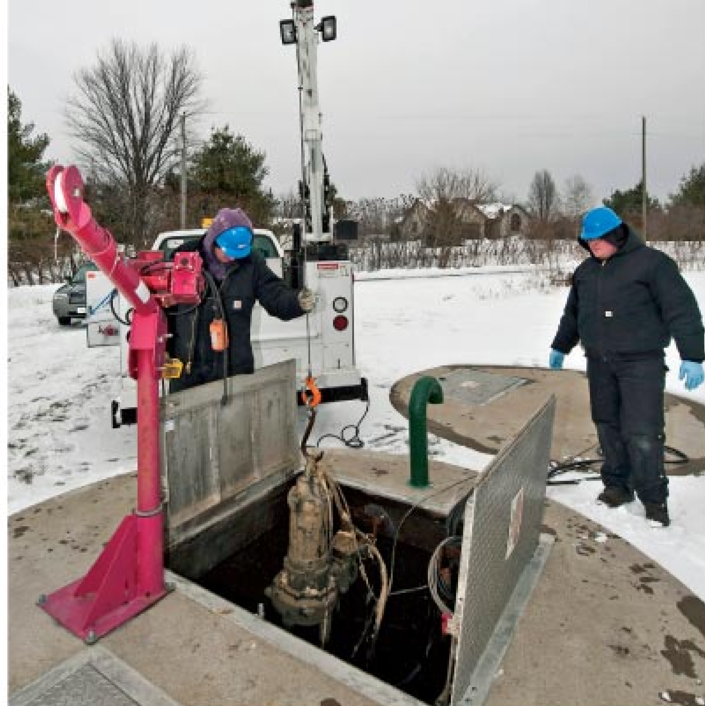
Tom Arey and Drew Lammers perform routine maintenance on an EBARA 20 hp submersible pump, one of two alternating pumps at a lift station serving a new subdivision in North Liberty.
