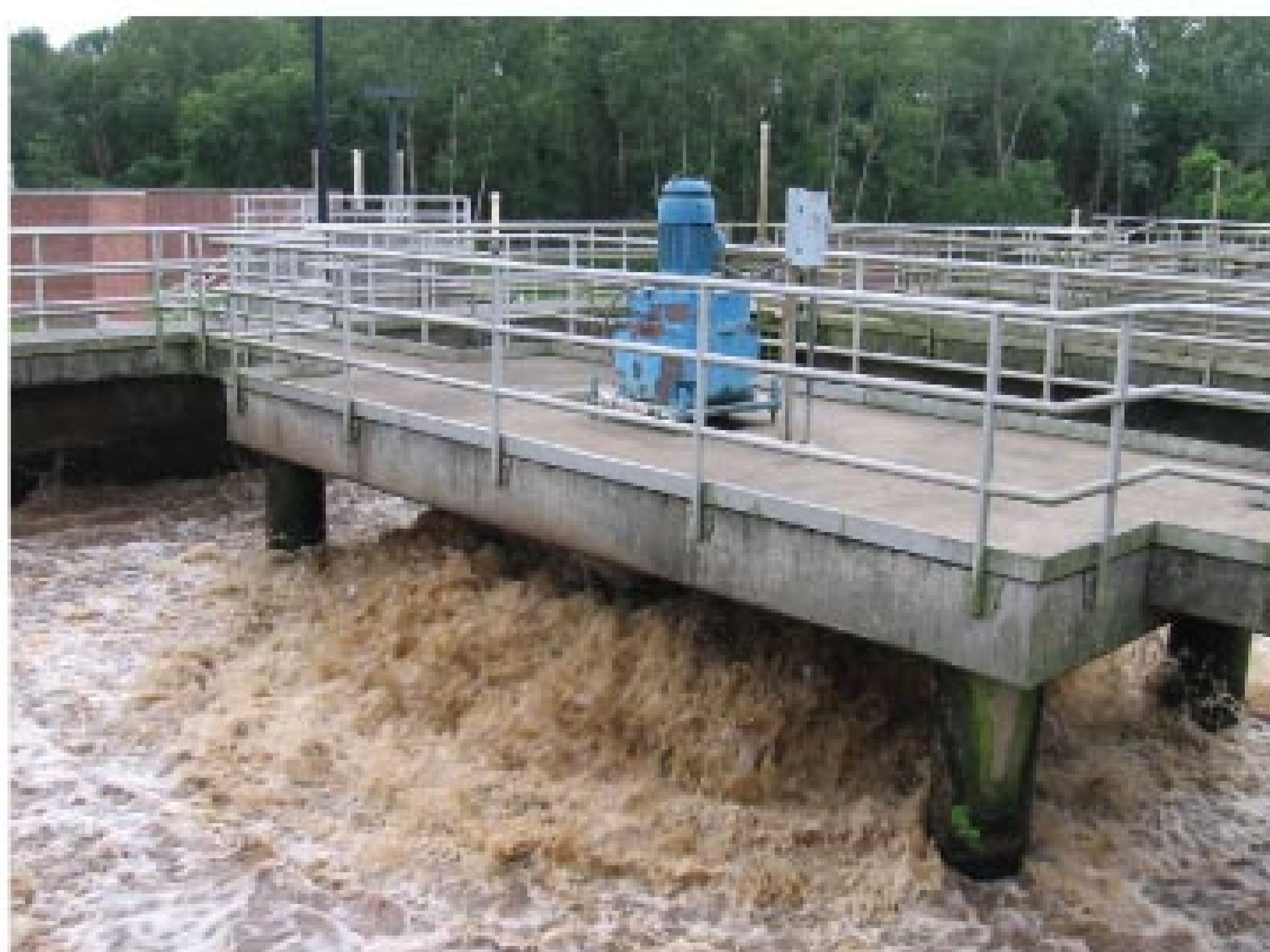
At the time of the upgrade, the plant’s mechanical aerators were more than 30 years old and badly needed replacement.
