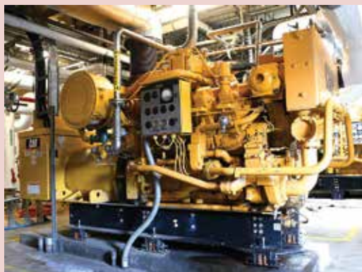
Two Caterpillar C3508 engine-generators fueled with biogas are part of a combined heat and power system that helps the Gresham (Oregon) Wastewater Treatment Plant achieve net-zero energy. The units provide a combine 800 kW capacity.
