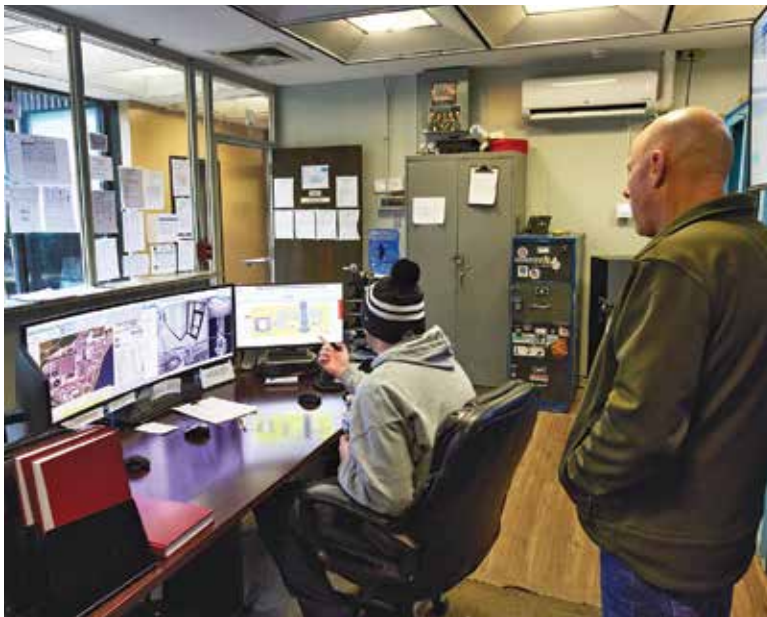
The plant's iFIX SCADA system was supplied by GE Digital.
