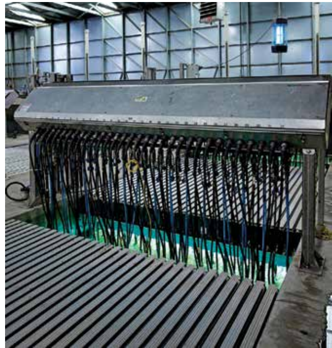
Treated water passes through a four-channel Trojan UV3000 Plus disinfection system before discharge to the Atlantic Ocean.
