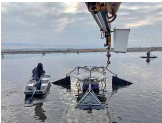
One of four SolarBee mixers being installed using a crane at the Grandview lagoon.
