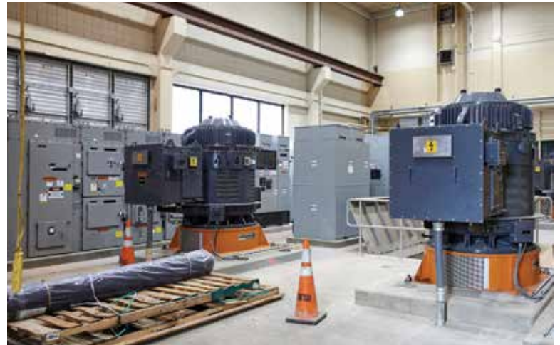
The pump room at the Bergen Point treatment plant includes pumps from Flowserve.
