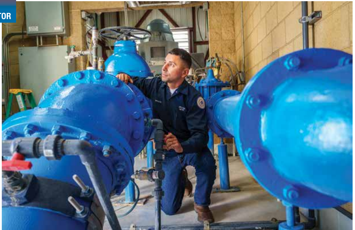
Horacio Palacios helps operate a water system that includes 10 booster stations, 13 storage tanks, 30 regulating valves, 30 wells and more than 600 miles of mains.
