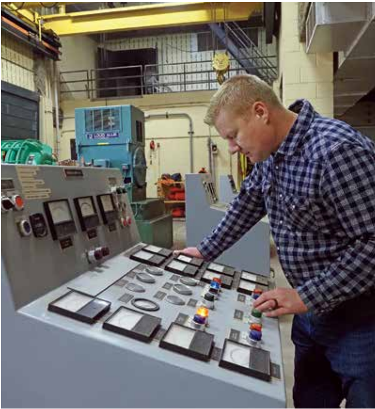
Huston is proud to work in an industry that is growing in sophistication as its professionals deal with increasingly complex and important issues. (Blower control panels from Hoffman.)
