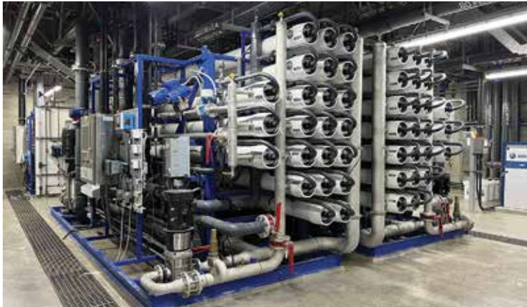
The reverse osmosis equipment at Santa Monica’s Sustainable Water Infrastructure Project is all underground (H 2 O Innovation).
