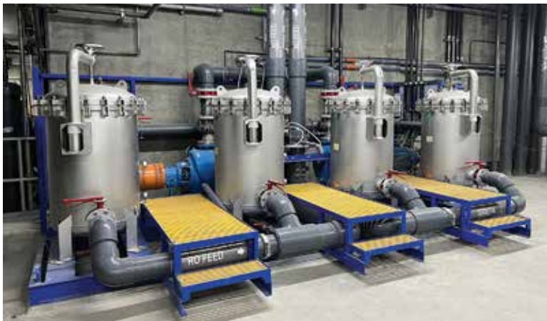
Cartridge filtration is part of the advanced water treatment process at the Sustainable Water Infrastructure Project (Harmsco).
