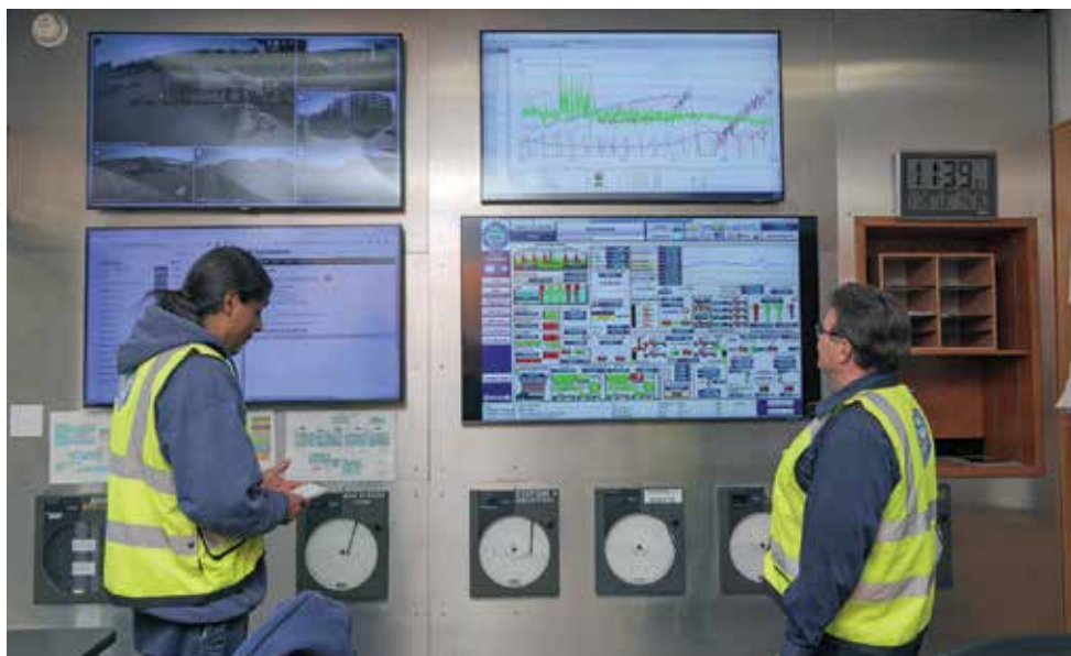
Manuel Dos Santos (right), had a significant role in developing the plant SCADA system, which was largely an in-house project.
