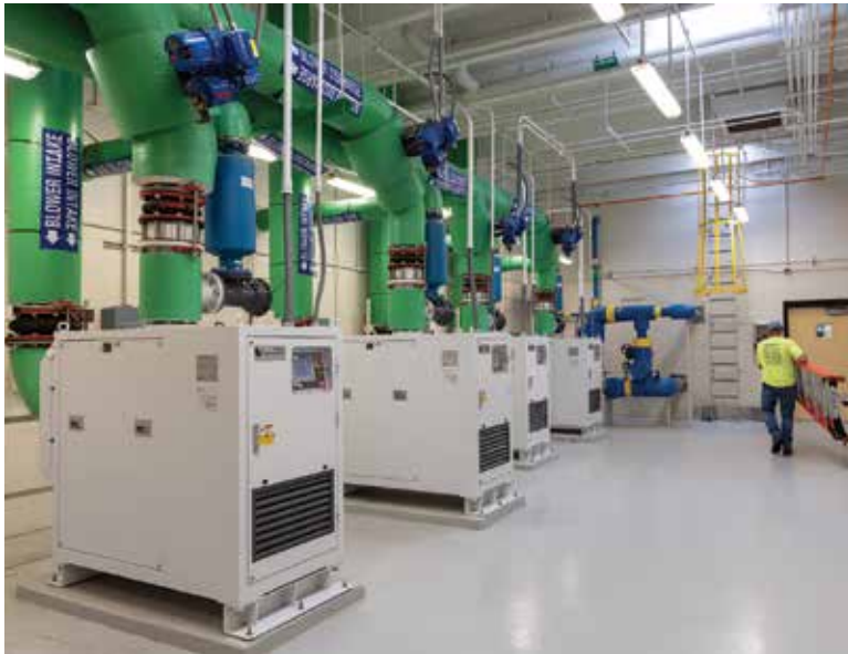
APG-Neuros NX100 turbo blowers at the The North Slope Wastewater Treatment Plant.
