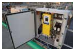
ChemScan mini Outdoor Enclosure from In-Situ
