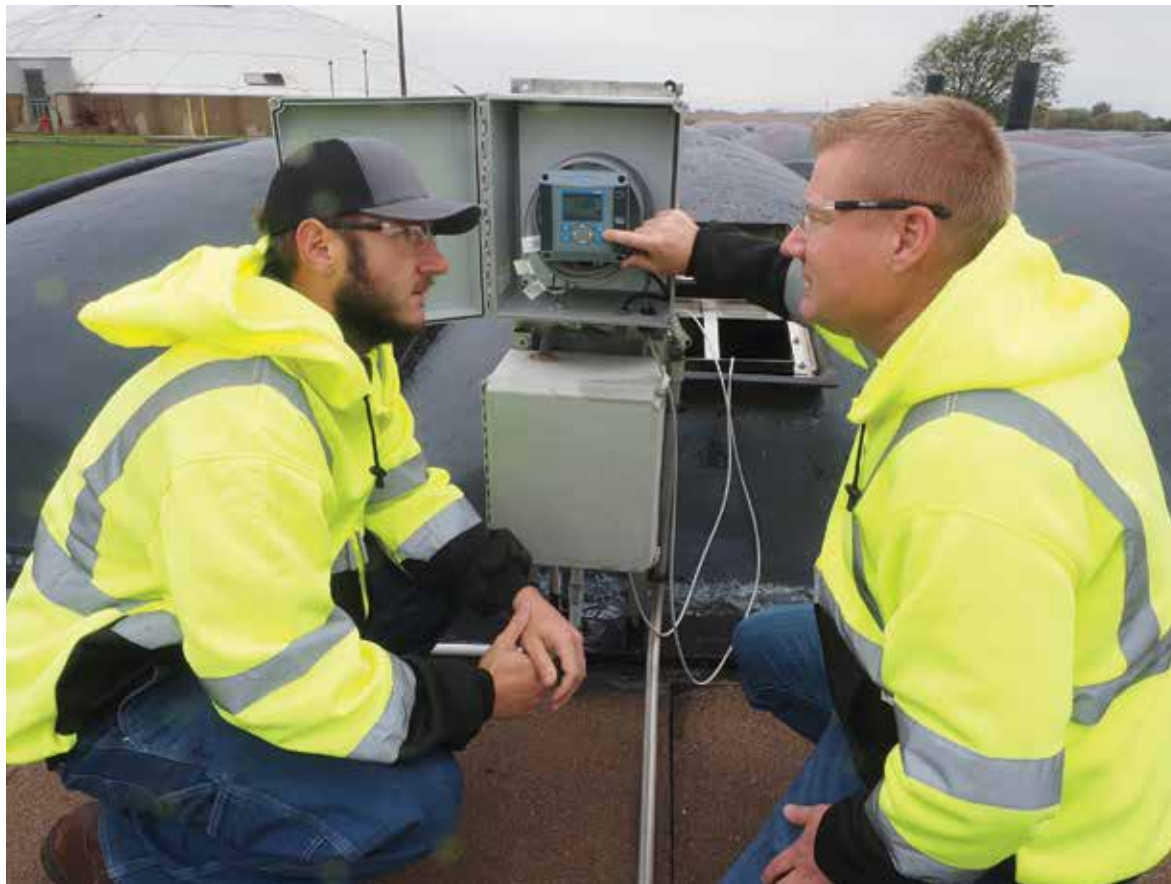
Huston, right, named Outstanding Rookie Operator of the Year by the Minnesota Wastewater Operator Association, works with Cavit Wobschall to calibrate dissolved probes using a Hach SC200 controller.
