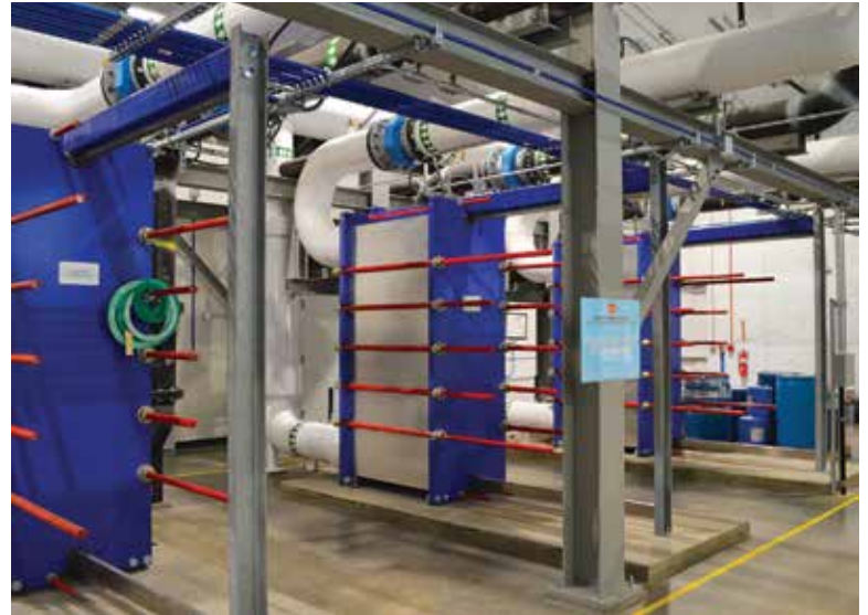
Inside the central utility plant, a wastewater stream diverted from a 72-inch sewer pipe goes through macerator pumps to remove solids, then through heat exchangers (Alfa Laval).
