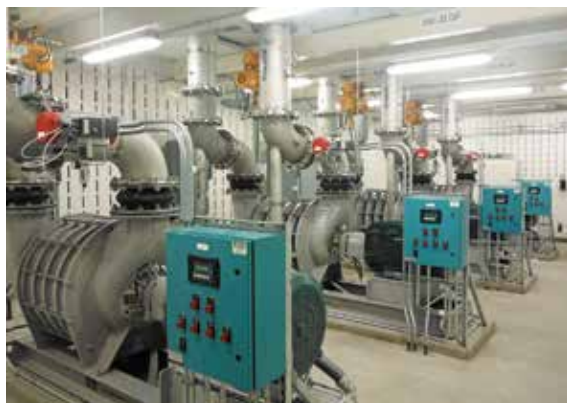
The Lake Stevens team controls effluent nutrients by shutting down the blowers to a lone aeration basin for most of the day.
