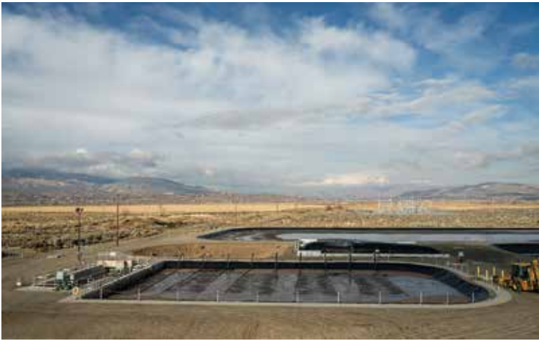
The Minden treatment plant has two basins designed to treat 0.9 mgd. Average flow is about 500,000 gpd.
