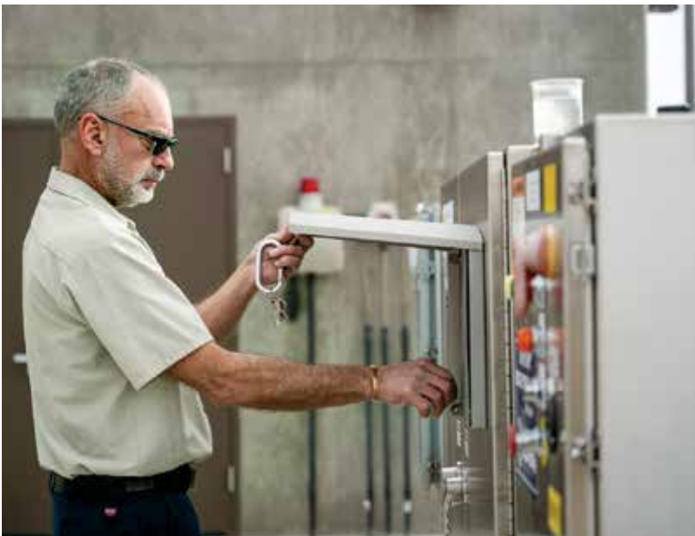
Michalak, at the control panel for the headworks (Lakeside Equipment Corporation), got a late start in the clean-water profession but has found it rewarding.
