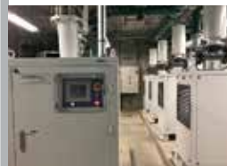
Advanced Aeration Control System from APG Neuros
