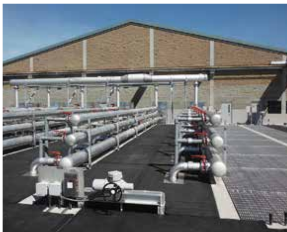
The pipe gallery at the Lake Stevens treatment facility.
