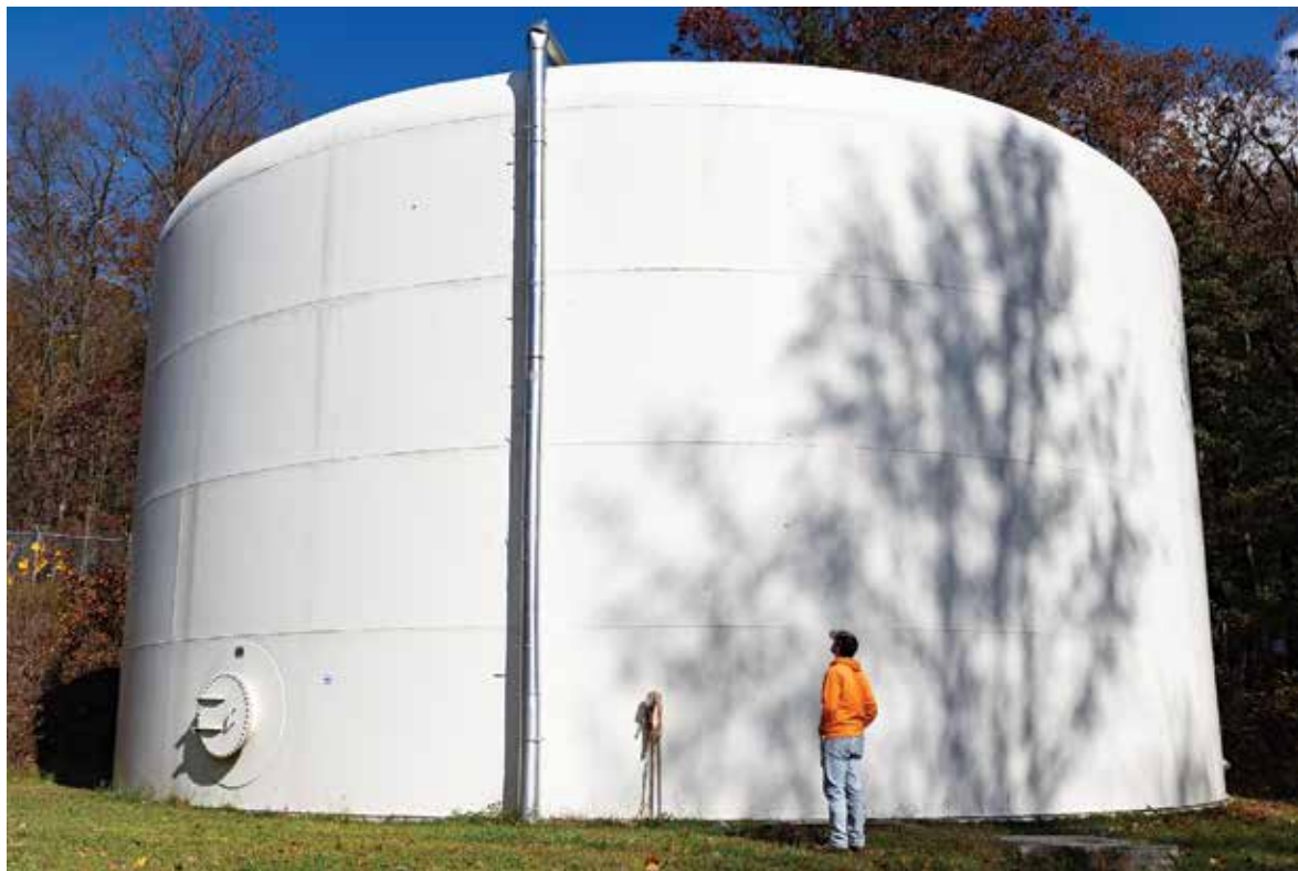
The Tower City Borough Authority draws from four deep groundwater wells. The system is rated to produce 250,000 gpd to serve about 1,200 connections.
