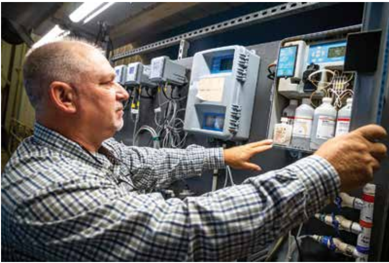
Ziegler, shown with an instrument bank that includes a Hach CL17 chlorine analyzer, leads a team at a conventional water plant built in 1988 and upgraded several times.
