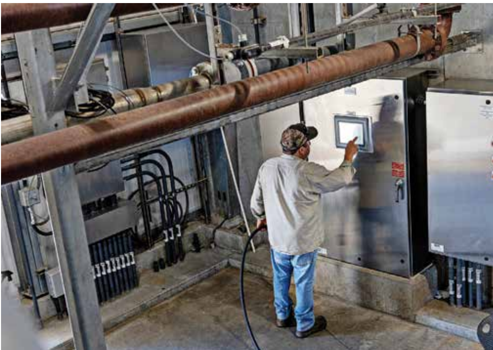
Paco Orona at the control panel for the FKCs screw presses, which dewater biosolids content to 15-29% solids.
