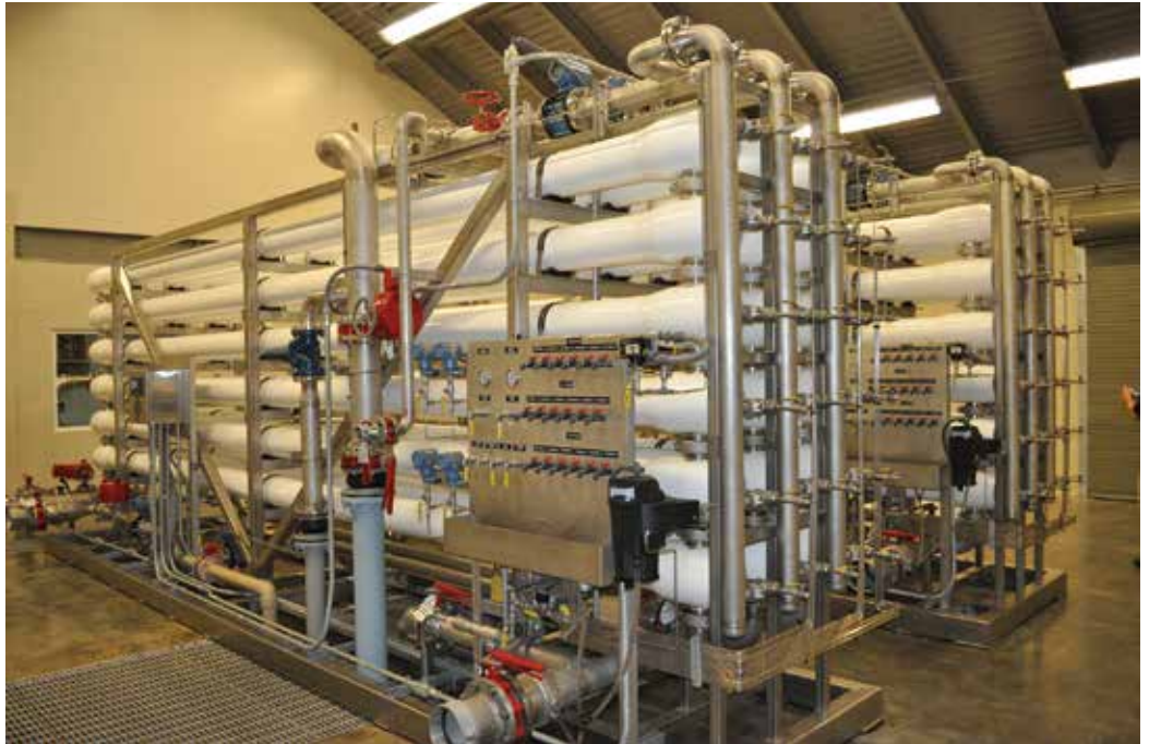
The main room inside the Dauphin Island reverse osmosis water treatment plant stays at 76 degrees without climate control.
