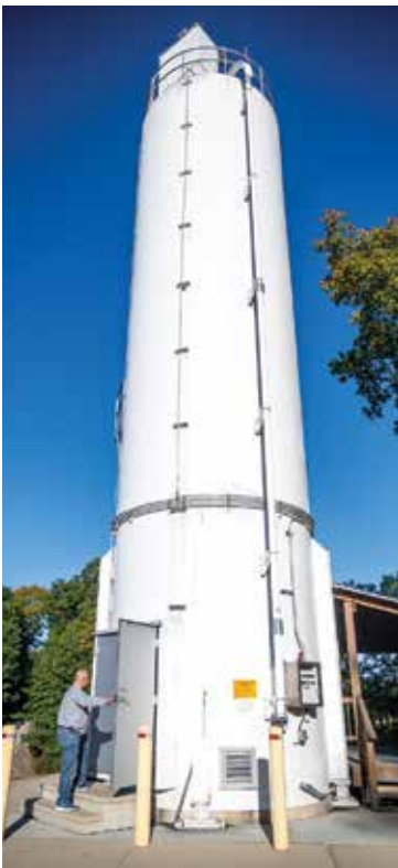
Ziegler checks the carbon feed silo system (MERRICK) at the water plant, which has a treatment capacity of 6 mgd and an average output of 1.6 mgd.
