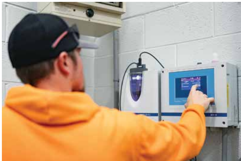
Tschopp calibrates the chlorine analyzer at Well 3 (Wallace & Tiernan DEPOLOX 5 analyzer from Evoqua Water Technologies, part of Xylem).
