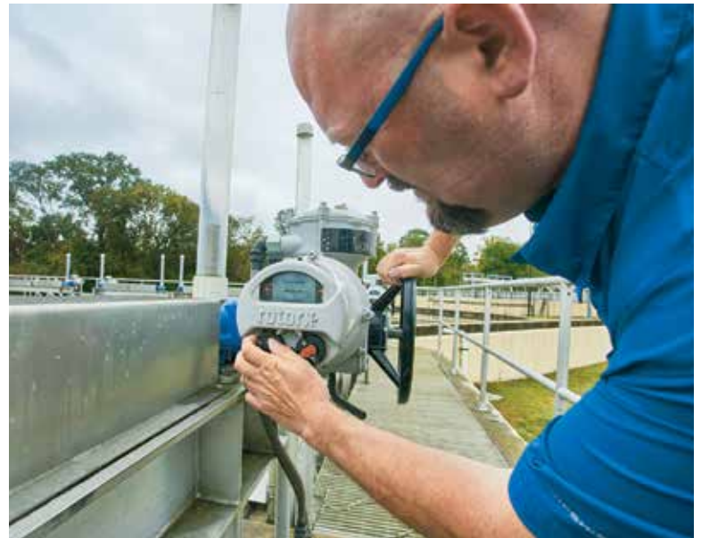
Boswell checks that the flocculation basins are operating properly (Rotork actuator).
