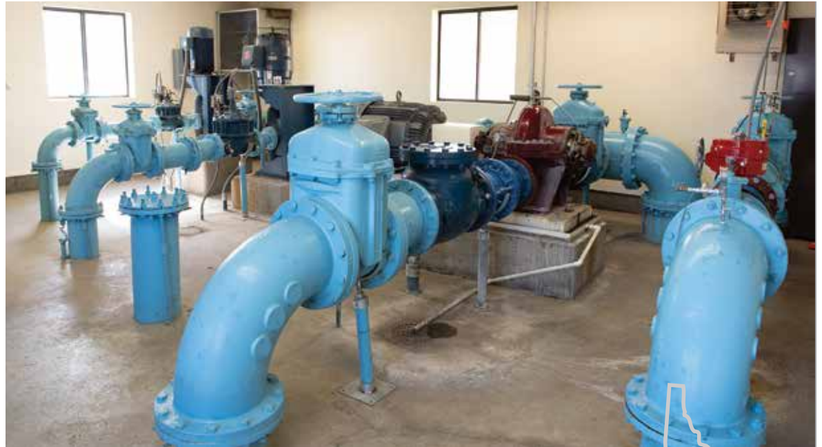
Gooding City Water Works main booster pump location (American-Marsh split case pump from Wilo).
