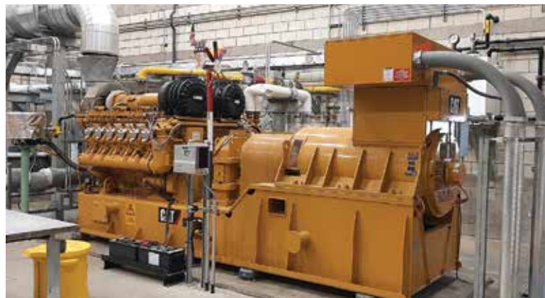
A 1.2 MW Caterpillar engine-generator drives the latest version of a combined heat and power system at the Willow Lake plant.
