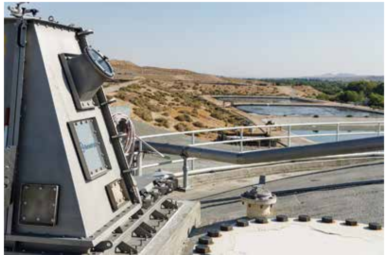
The view from atop one of the authority’s digesters, using Anaergia’s Omnivore technology.
