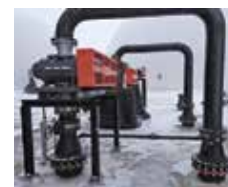
Aeration Blowers from TMC Fluid Systems
