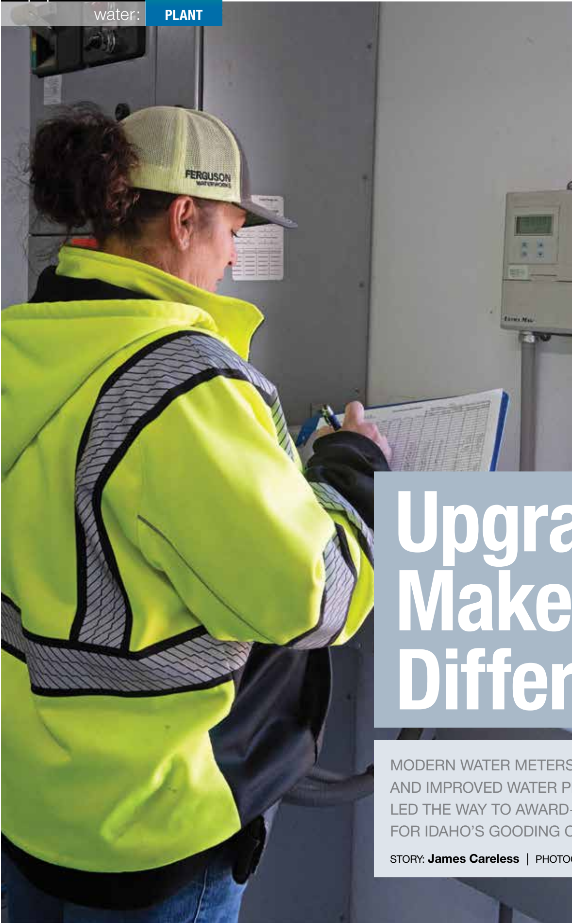
Pam Childs, water/wastewater operator, performs daily checks and testing on the Ultra Mag wastewater flowmeter (McCrometer) at the Gooding City plant.
