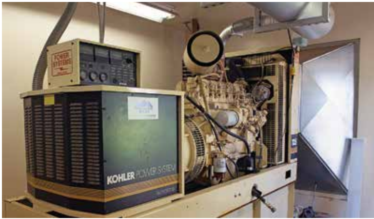
A Kohler generator provides backup power for the Gooding plant's main booster pump.
