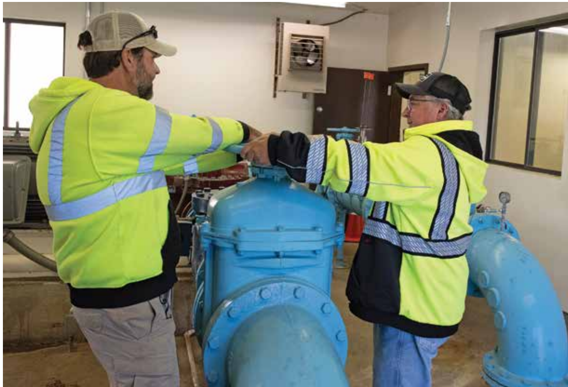
Gooding City Water Works staff members Joel Eilers (left) and Paul Childs perform daily checks and testing at the plant, which produces 200,000 gpd to 2.4 mgd.
