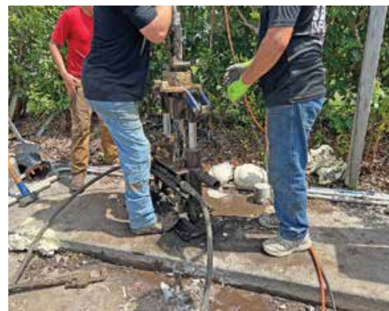
DHIG technology proved beneficial on projects in Sarasota and Hillsborough County in Florida.
