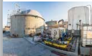
Omnivore anaerobic digester from Anaergia
