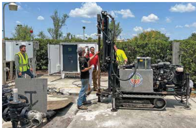
Grouting material can be injected from a lateral point and so prevent interference with nearby project activity, saving time and cost and limiting environmental impact.
