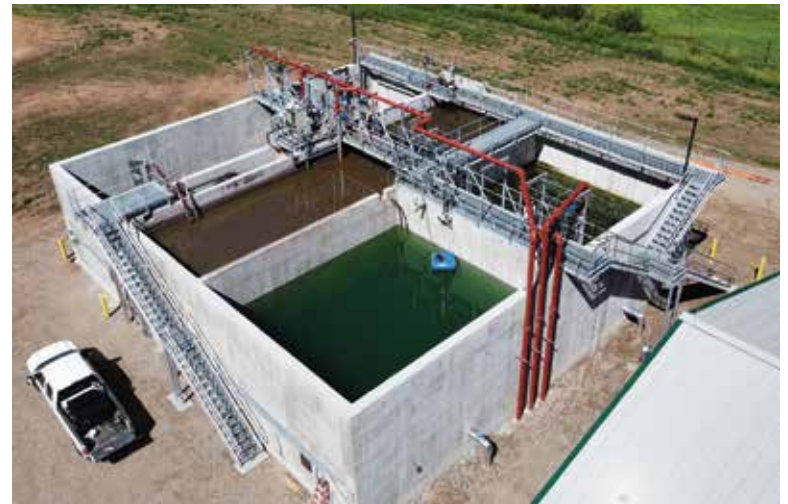
The BIOCOS process is a hybrid activated sludge system in which all mixing and recycling are driven by blower air, significantly reducing energy usage.
