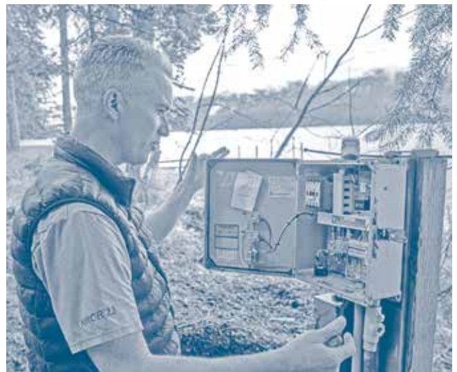
Larry Peterson puts a zip tie on knife switch in a lockout safety procedure on a pump control panel from Orenco Systems.
