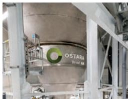
Ostara Pearl system from Evoqua Water Technologies
