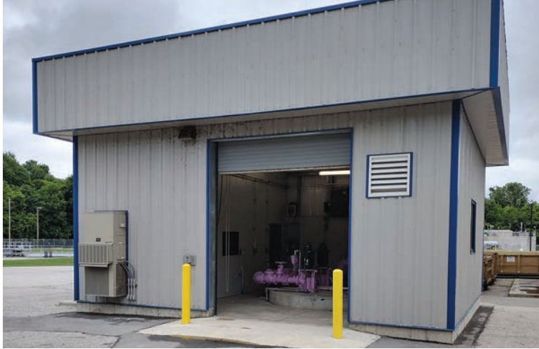
A new pump station houses pumps for reuse and cleanup water at the Lynn Lane Wastewater Treatment Plant.
