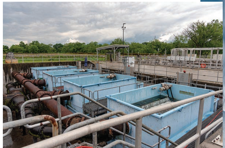
Tertiary filters at one of the Hallsdale-Powell Utility District’s two wastewater treatment plants.
