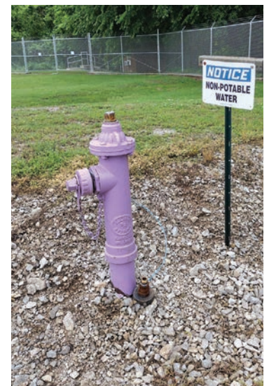
RIGHT: Hydrants around the wastewater treatment plant in Broken Arrow, Oklahoma, are painted purple to indicate reuse water.
