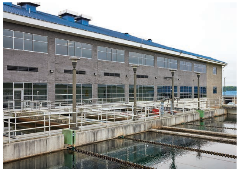
The treatment center at The Henry County Water Authority.
