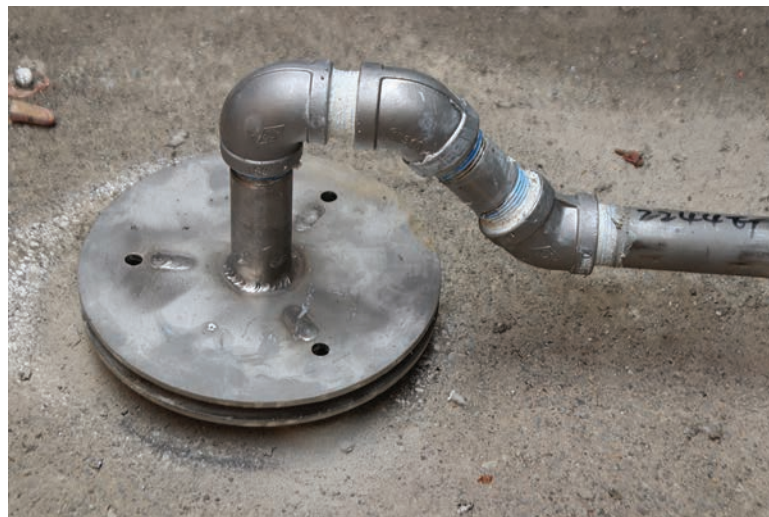
Bubble-forming plates help generate large bubbles that mix the anoxic zones in the Richmond treatment plant's first-stage aeration basins.
