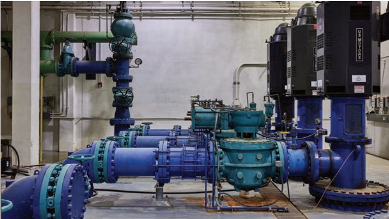
The high-service pump room at The Henry County Water Authority uses Goulds turbine pumps.
