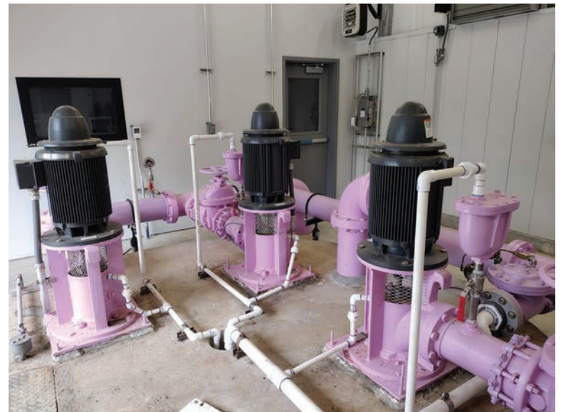
ABOVE: Inside the pump station that handles effluent for reuse. The plumbing is painted in the signature purple for recycled water.
