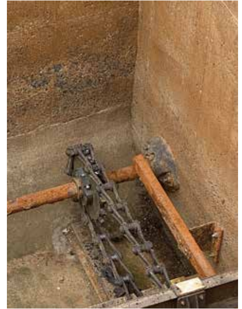
A close-up view of the clarifier mechanism's fiberglass-reinforced plastic chain.
