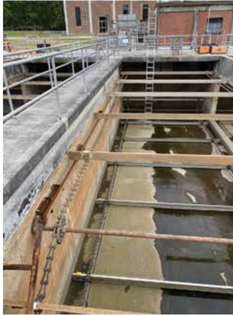
A rake in the clarifier at the Durham treatment facility. The wastewater has been drained to enable maintenance.
