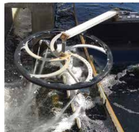
Automated algae control systems, like the WeirWasher cleaning system, can dramatically improve safety and efficiency.
