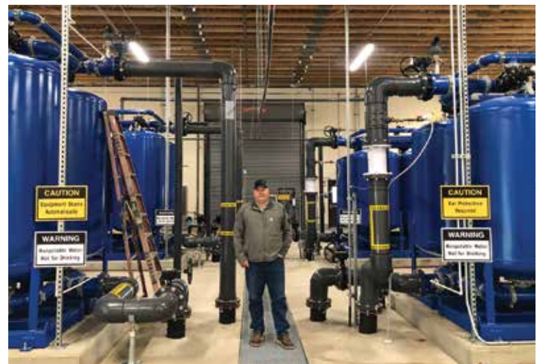
Eric Klann, Prineville city engineer and public works director, inside the Prineville Water Treatment Plant, which has a capacity of 3 mgd. In summer this capacity is augmented by an aquifer storage and recovery system.
