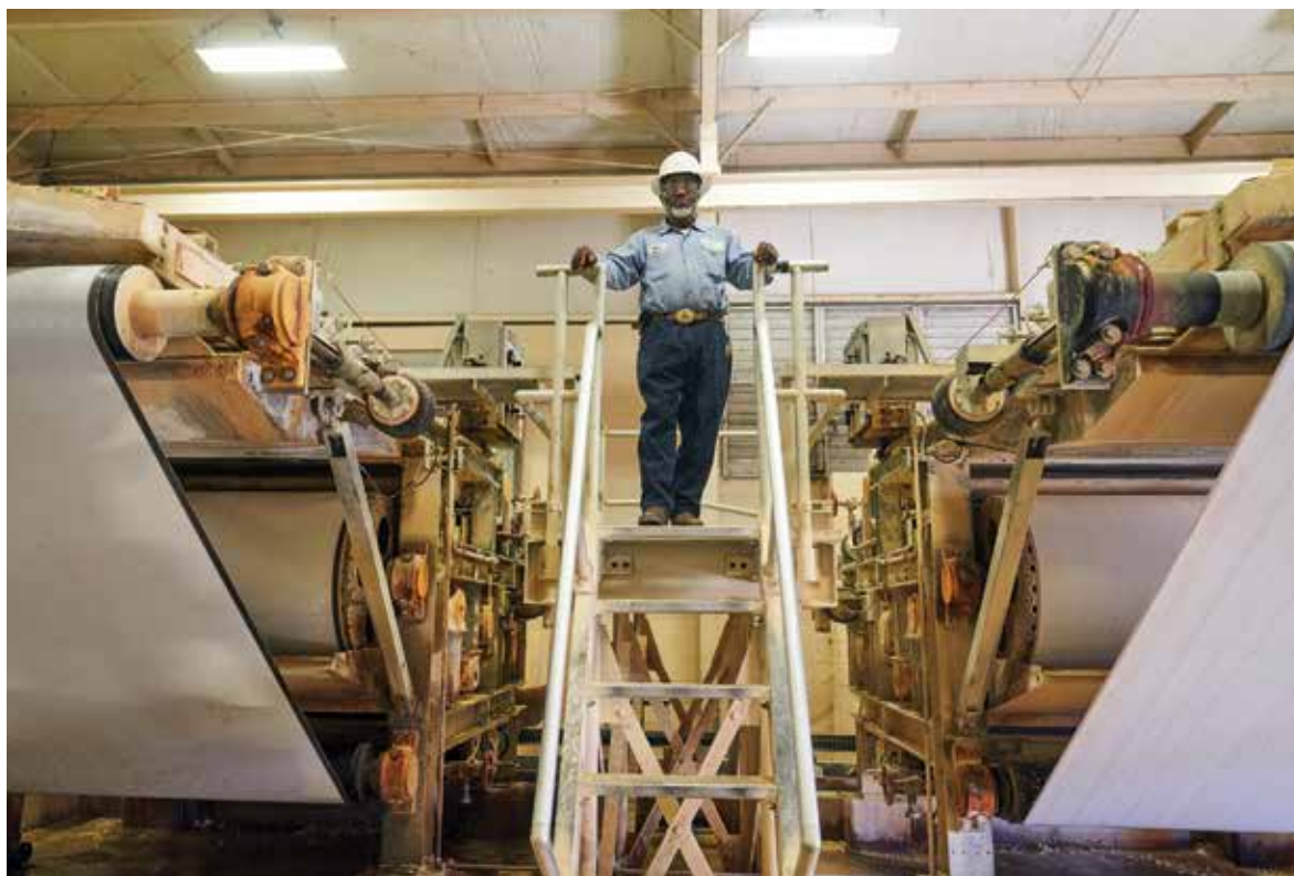
Willie Flagg with the plant's Andritz belt presses. Dewatered biosolids are sold to farmers as fertilizer and soil conditioner.
