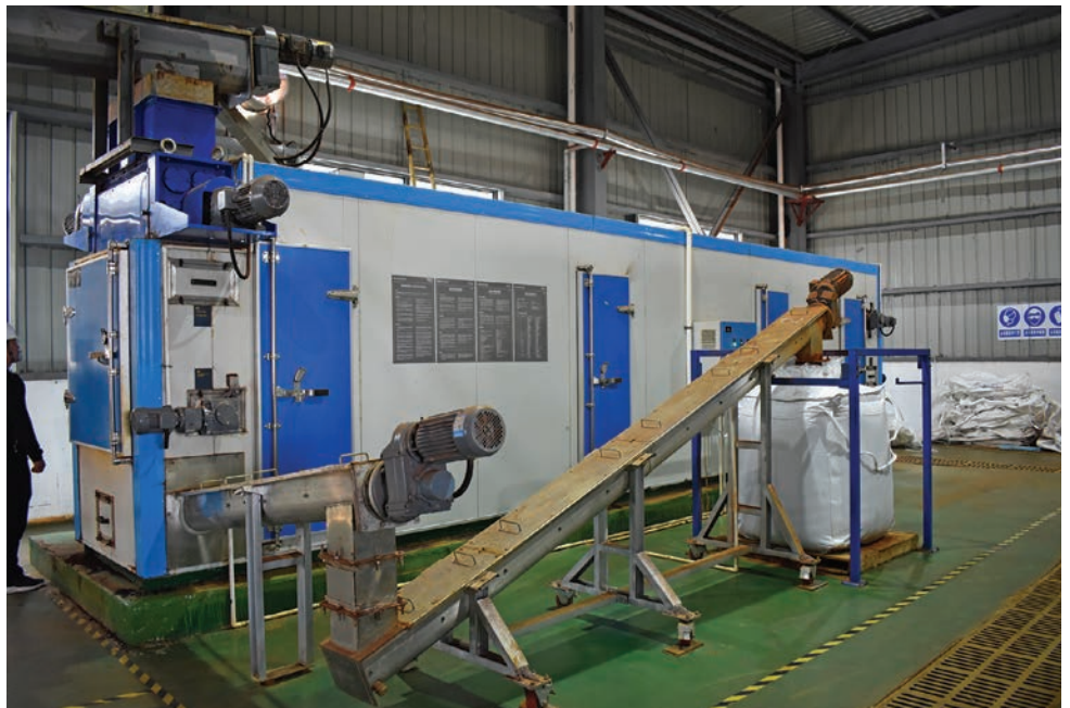
A Shincci dryer transforms wet cake into a Class A biosolids in about four hours.
