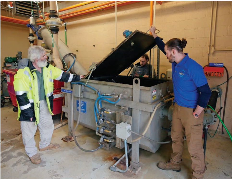
Checking the Complete Plant system (Lakeside Equipment) are, from left, Kendall Chamberlin, Allen Carpenter and Aaron Krymkowski.
