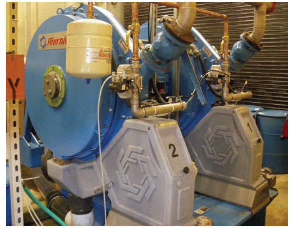
Biosolids are dewatered to 33% solids on this Fournier rotary press.
