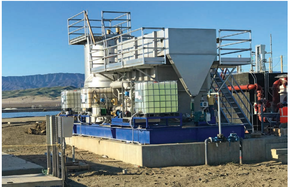
The skid-mounted Suspended Air Flotation unit (Heron Innovators) creates fine bubbles using a froth generator.
