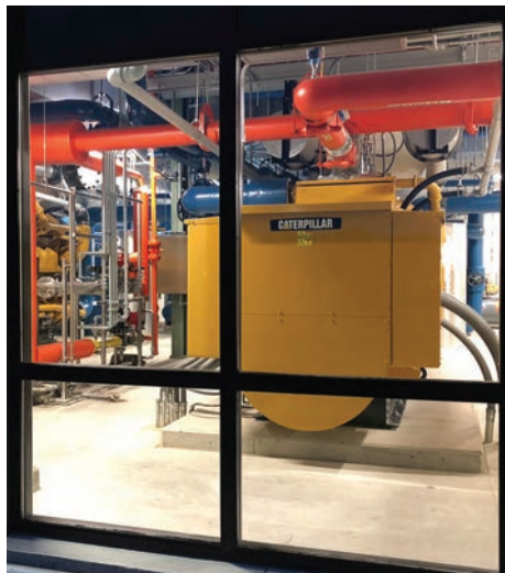
The combined heat and power system is driven by two Caterpillar 3520C engine-generators.
