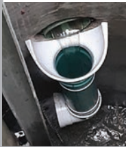
Lift Station Inside Drop from RELINER/Duran
