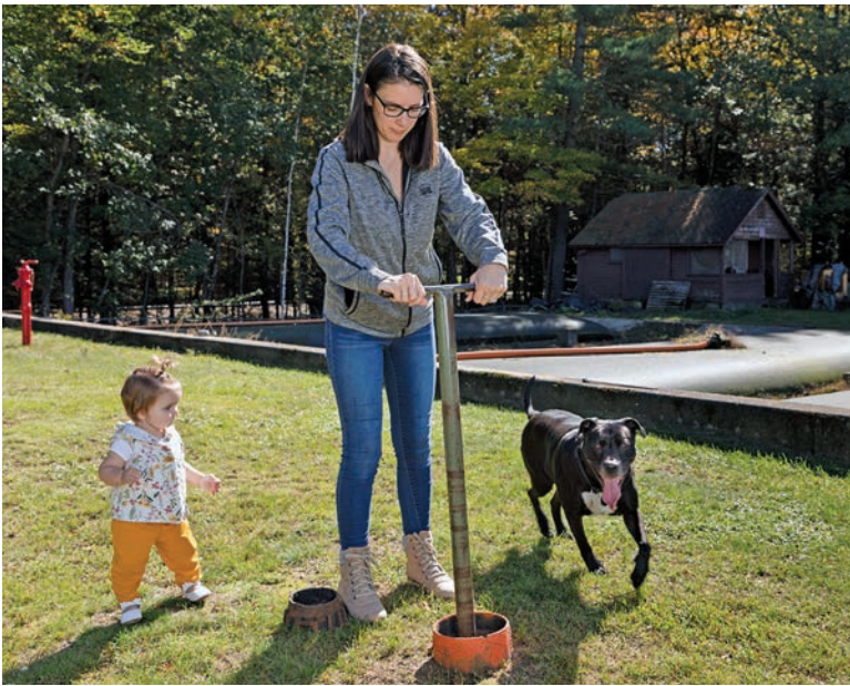
Hillary Welch opens a waste activated sludge valve to feed sludge holding bags. Her daughter supervises.
