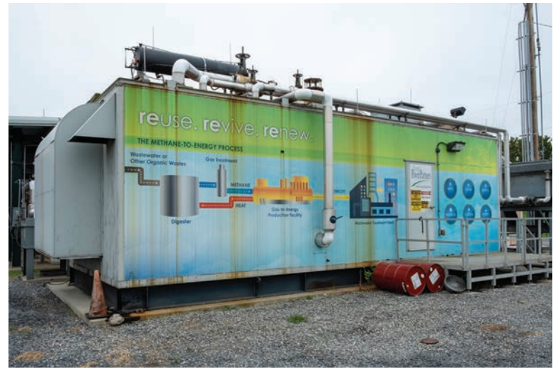
Kline's Island has a biogas-to-energy system that can provide about 50% of the plant's electricity.
