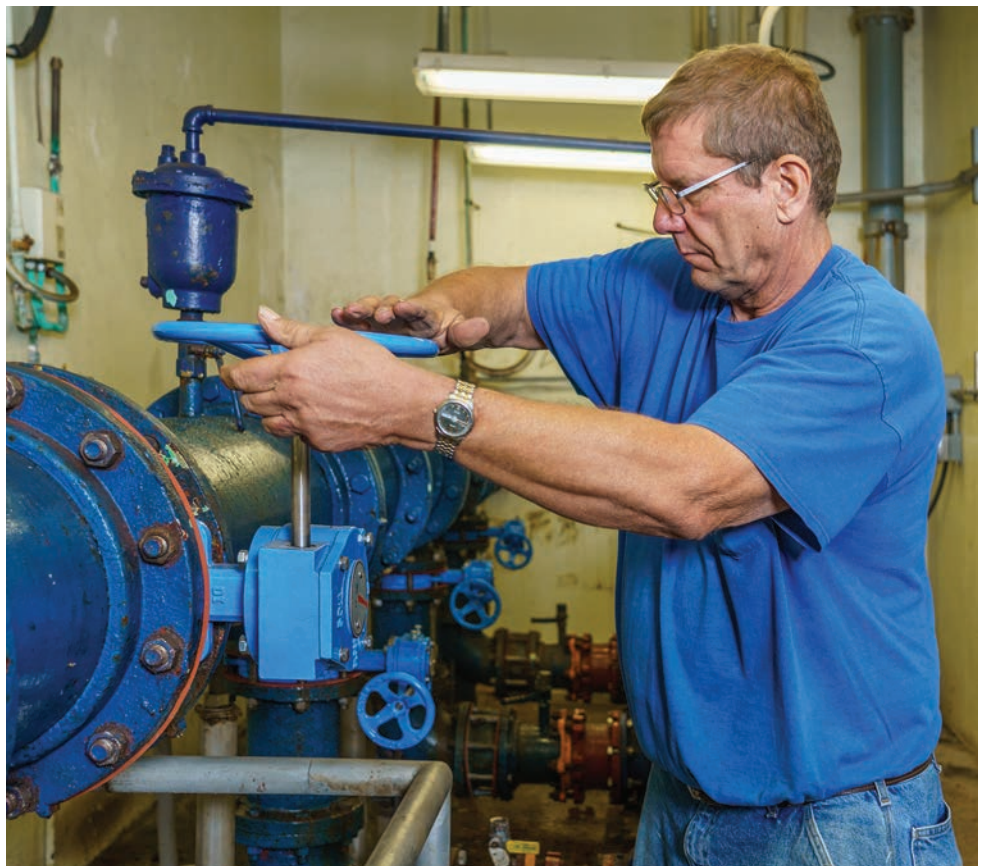
Tournade, shown working one of the newly installed valves (Henry Pratt) in the pipe gallery, has helped improve plant reliability and reduce after-hours service calls.
