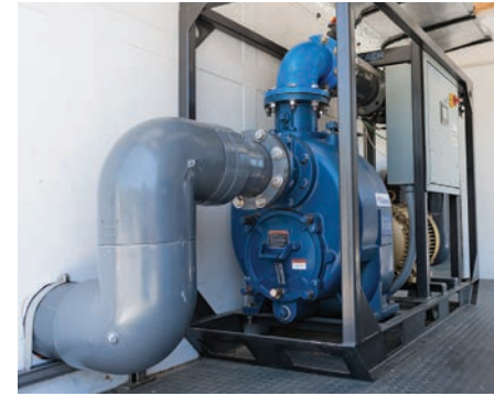
The interior of the Moleaer on-demand nanobubble generator trailer system.
