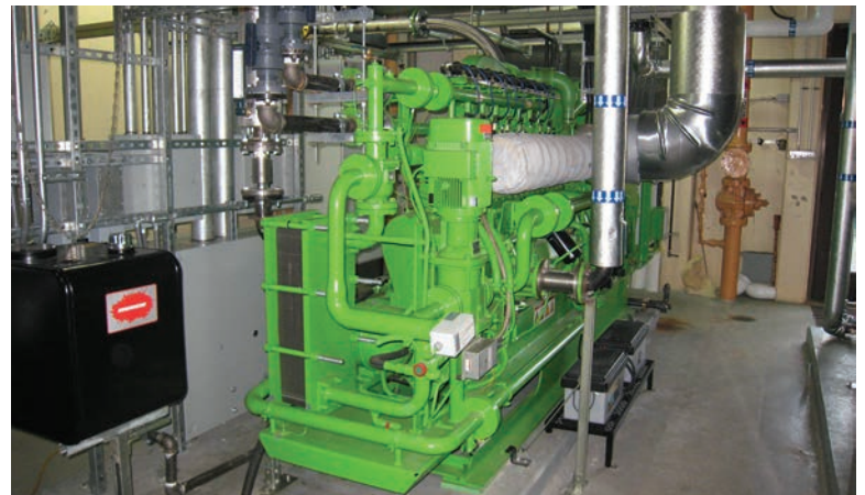
The Jenbacher (GE) engine has powered the cogeneration system at Budd Inlet plant since 2009.
