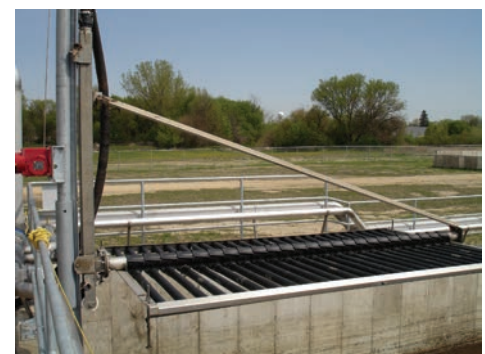
All components are accessible from the side of the basin for ease of maintenance.
