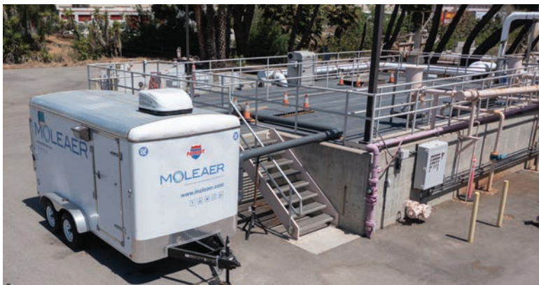
The on-demand nanobubble treatment system underwent a successful pilot test, documenting that the technology could improve treatment efficiency and reduce energy costs.
