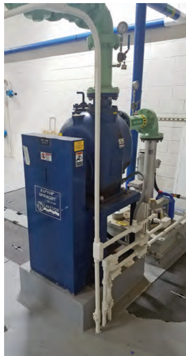
The SpiraGrit system (Lakeside Equipment) captures grit particles in a flat-floor circular upper chamber.
