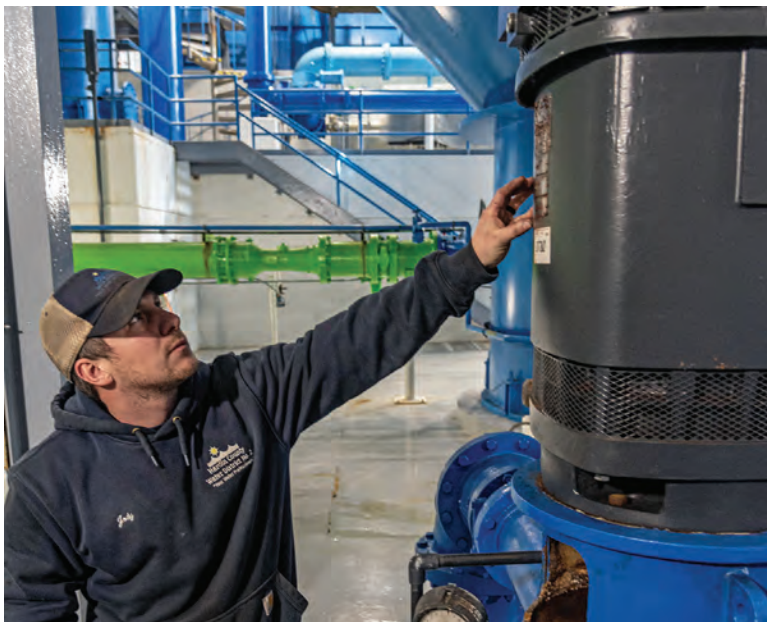
Jody Nalley, maintenance technician, checks the packing motor (Nidec) and oil levels on a Peerless vertical turbine pump (Grundfos).
