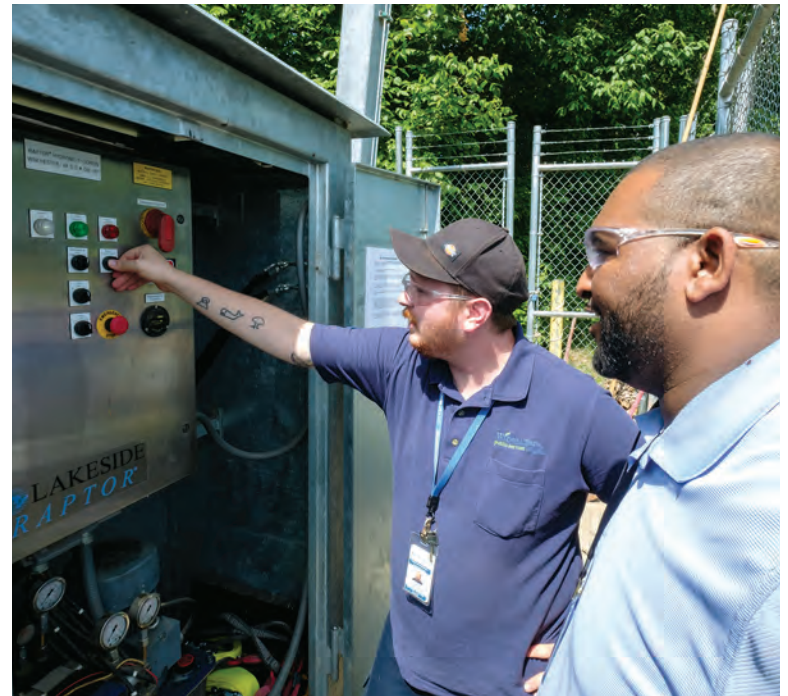
The facility uses an automated Raptor screening system (Lakeside Equipment).
