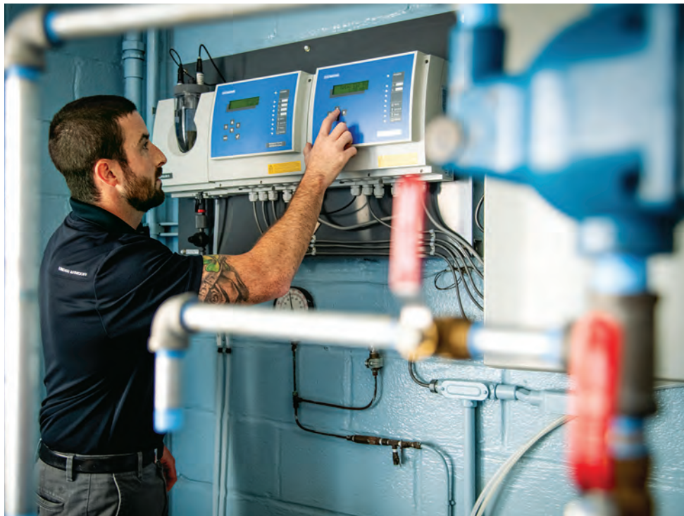
Botterman, water and sewer superintendent, checks the village's water quality utilizing Wallace & Tiernan analyzers and controllers (Evoqua).
