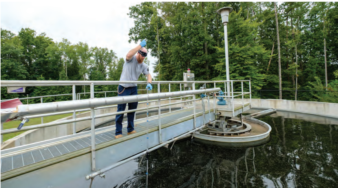
The plant has two final clarifiers and two cloth filters that put the finishing touches on water for reuse or discharge.
