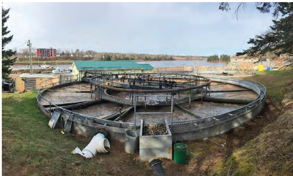
Influent arrives at the Montague return activated sludge package plant.
