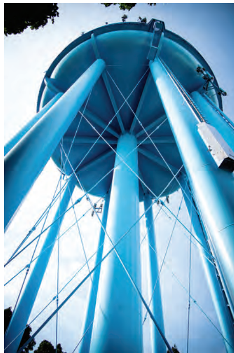
One of Mount Prospect's seven water storage tanks, which as of 2019 had all been rehabilitated.
