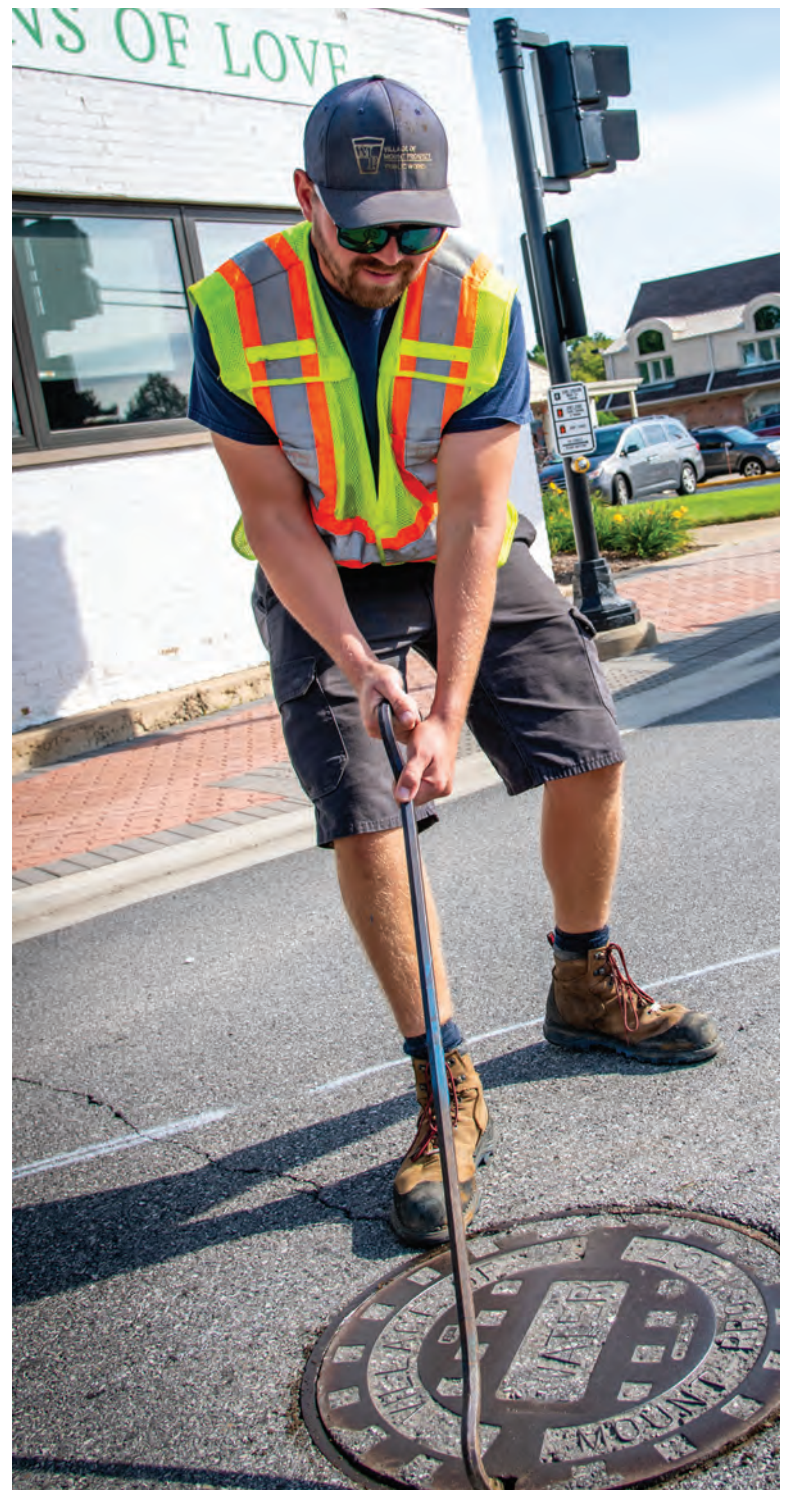
Jake Sprow removes a cover for valve exercising in anticipation of their water main lining project.
