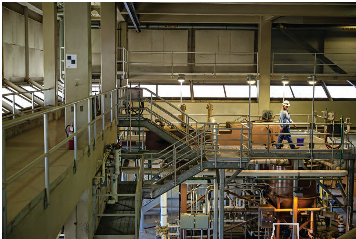
Tarantino inspects the furnace facilities within the Central San solids building.
