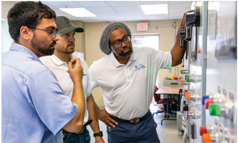
From left, Raymond Perez, wastewater operator; Richard Britton, operations supervisor; and Clifford Creeks Jr., supervisor IV/operations, monitor the bar screen control panel for alarms.
