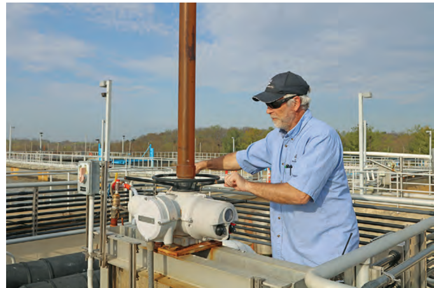
Jayson Warren, water reclamation operator, raises the level of one of three equalization basins during a high-flow demonstration.
