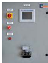
InGenius control panels from AdEdge Water Technologies
