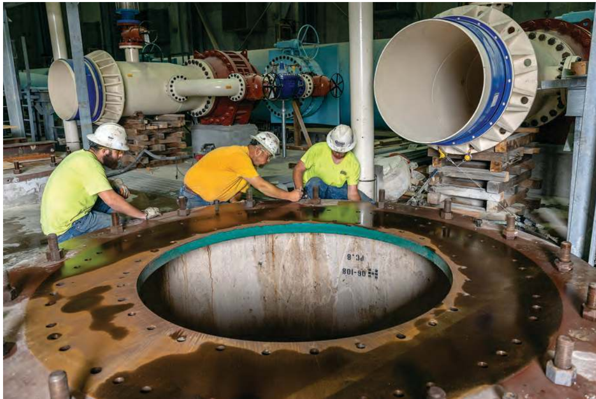
Garney Construction workers install two pumps (Odessa Pumps) for the conveyance station.
