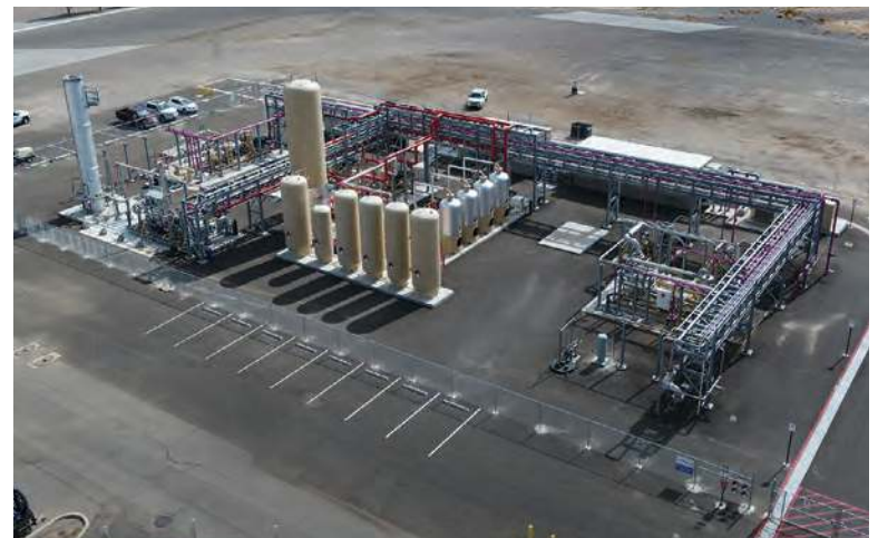
A renewable natural gas plant operated by Ameresco is on the site of the 91st Avenue Wastewater Treatment Plant in Phoenix.
