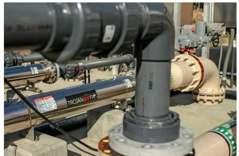
Effluent is disinfected in a TrojanUVFit system.
