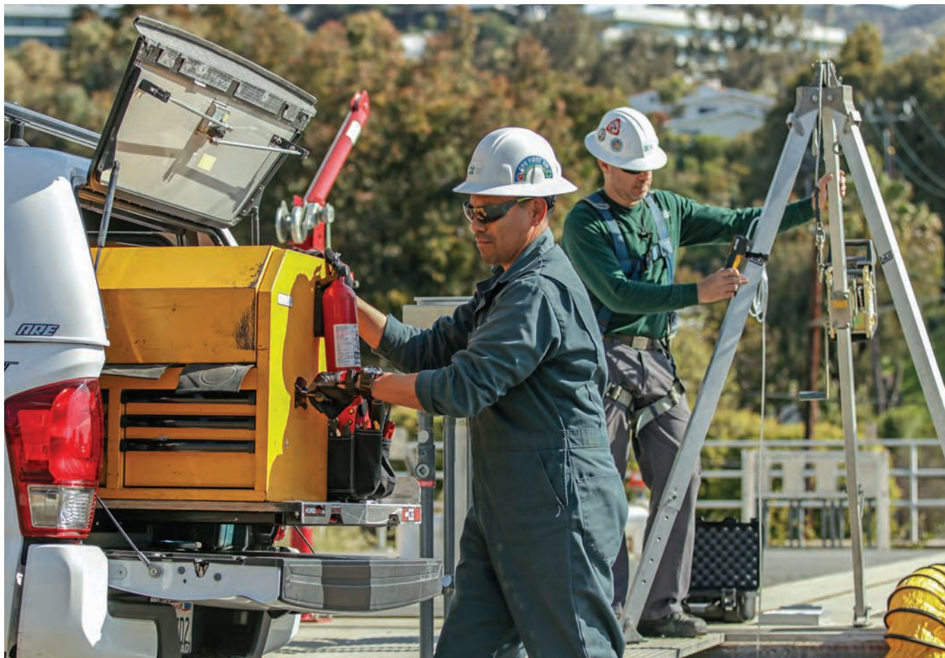
Carlos Alvarez (left) and Golan Kfir perform routine maintenance at the treatment facility.
