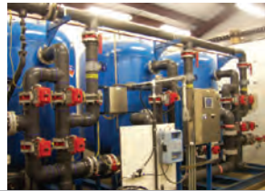
Biotta biological filtration system from AdEdge Water Technologies
