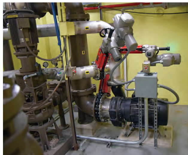
The 49 hp centrifugal Landia chopper pump (on right with knife valves) recirculates sludge from the digester.
