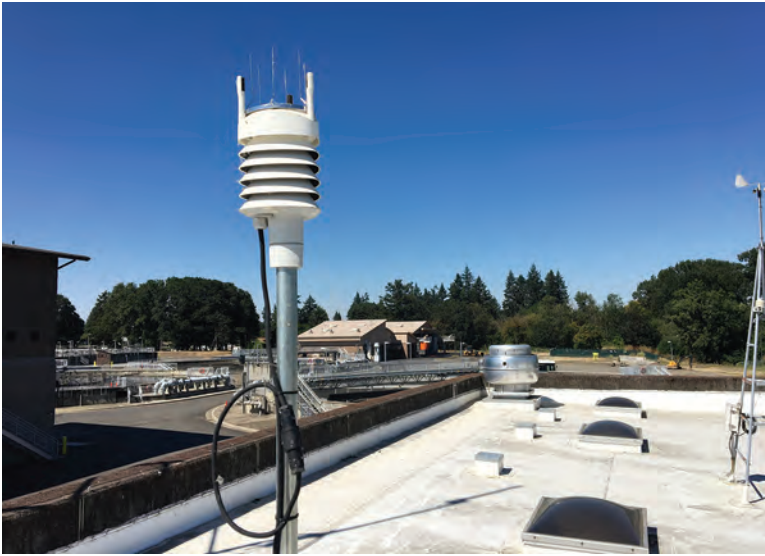
The water reclamation facility in Albany uses an Orion Weather Station all-in-one sensor from Columbia Weather Systems to monitor wind speed and direction with ultrasonic technology, as well as rainfall, temperature, humidity and barometric pressure.
