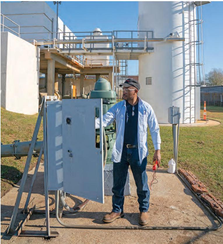
Albert Edmonds, plant technician, checks an electrical panel at the South Water Treatment Plant.
