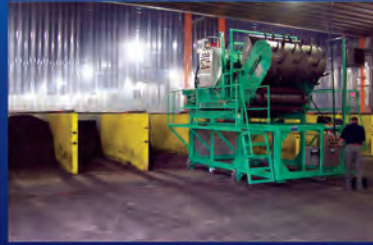
Agitated and Aerated In-vessel type Composting System (ICS)
