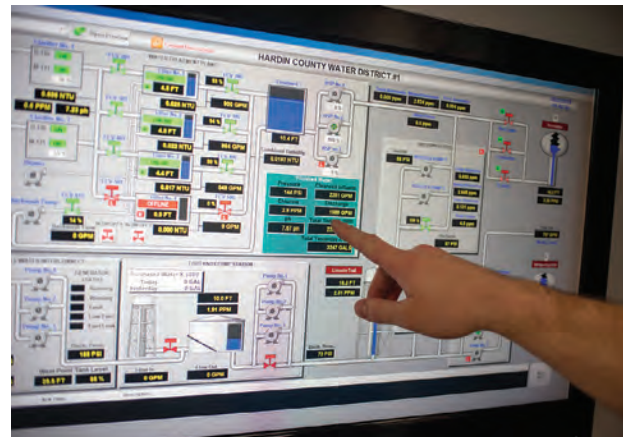
A SCADA system helps operators keep tabs on plant operations.
