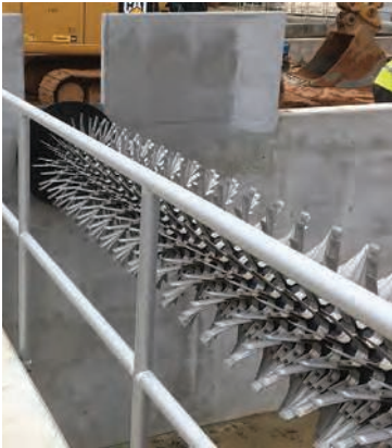
The Magna Rotor aeration system (Lakeside Equipment) provides precise oxygen input to the biological treatment process.
