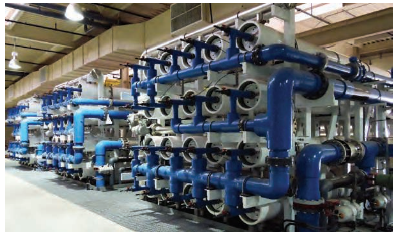
Scottsdale’s 20 mgd advanced water treatment includes this reverse osmosis system.
