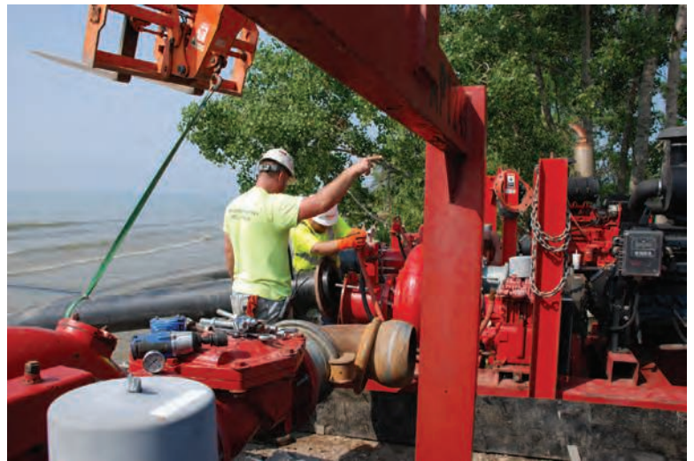
Tim Campbell (left) signals forklift driver Mark Bernal to keep retracting the boom as Erick Halaburt helps align the first rod in the 14-inch pump flange.
