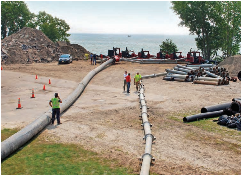
Cleaning the pipe is underway as the dive boat motors out to the intake riser.
