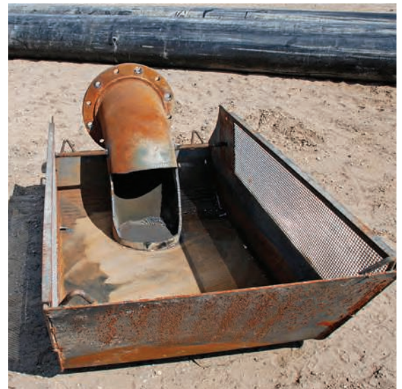
The 72- by 36- by 24-inch-deep sleds helped anchor the HDPE pipes in water. Solid bottoms and elevated elbows eliminated drawing sand and sediment into the pipes.
