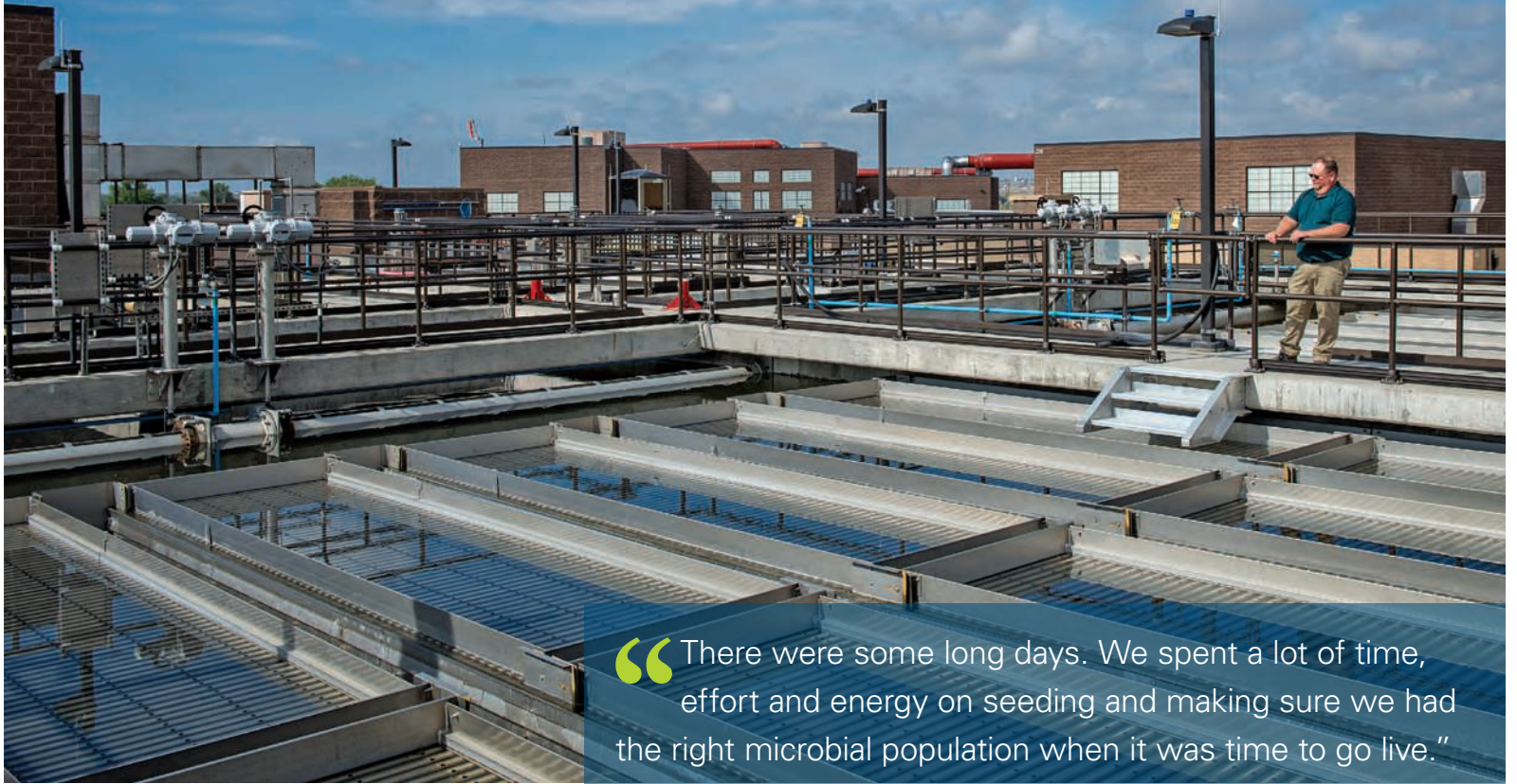
The tertiary floc sedimentation facility at the Northern Treatment Plant.
