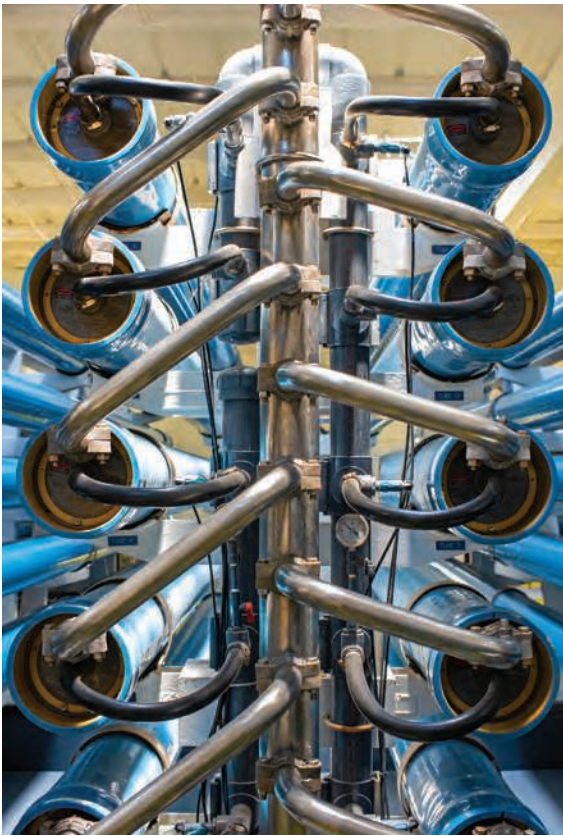
High-pressure pumps push water through the RO membranes. Each blue tube contains six membranes.
