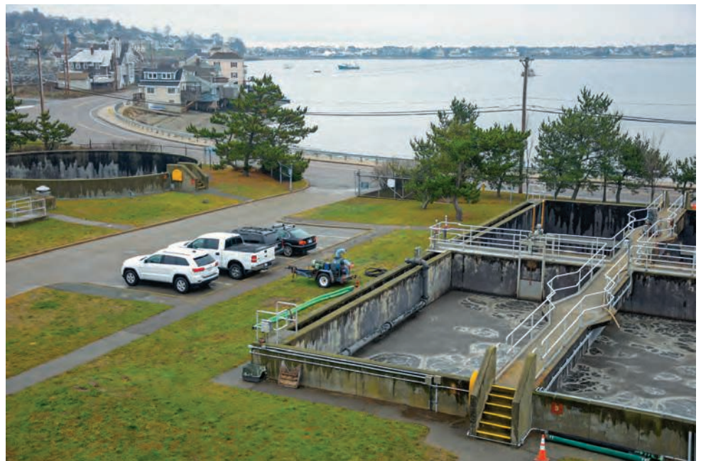
The Hull facility is a conventional activated sludge plant with a design capacity of 3.07 mgd. The collections system serves about 4,000 residential and business connections.
