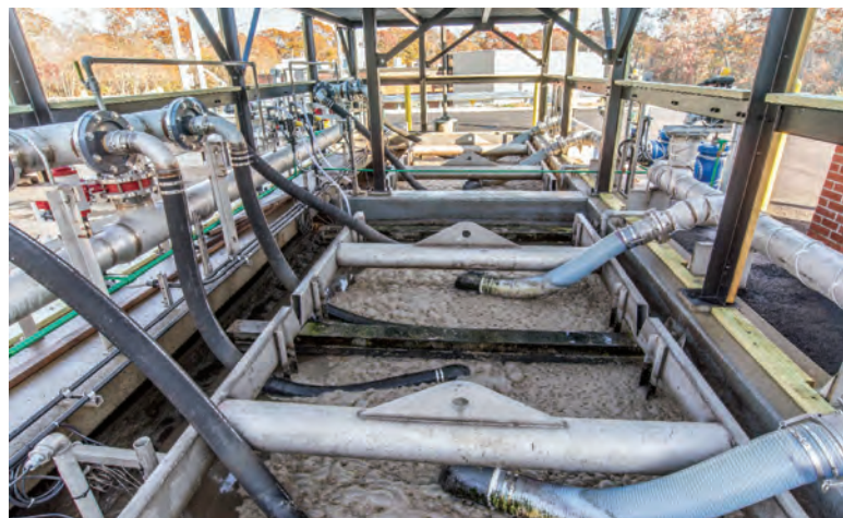
The effluent at the Riverhead facility undergoes membrane microfiltration as part of the water reclamation process (Koch Membrane Systems).
