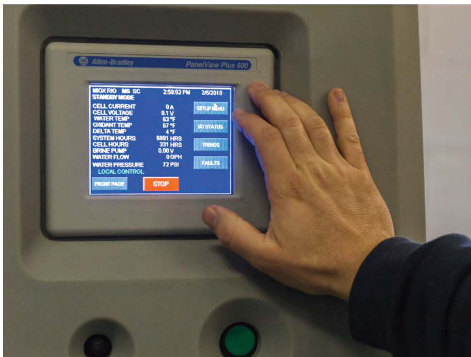
The Prestonsburg plant uses a MIOX system for disinfection in place of chlorine, using an Allen-Bradley PanelView Plus terminal (Rockwell Automation).
