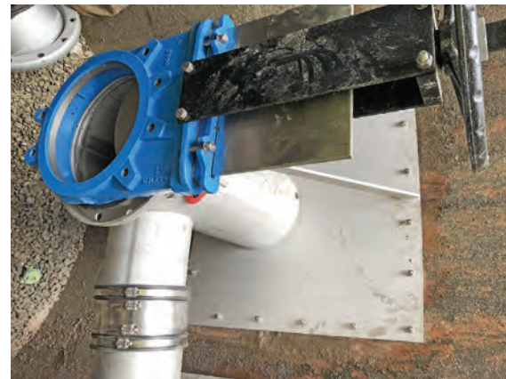
Flanges connect the lift station inlets directly to the pumps.
