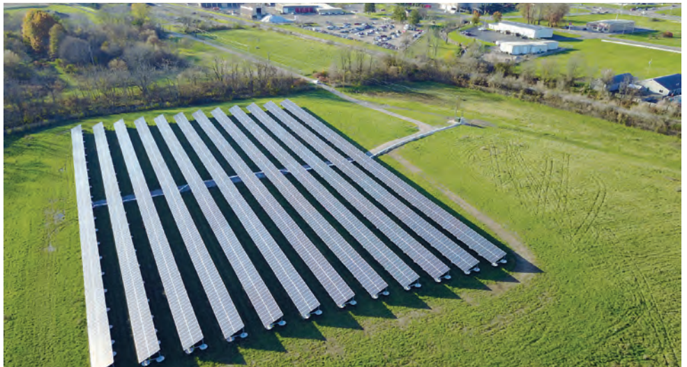
The solar array includes 3,312 panels and occupies 5 acres. AEP OnSite Partners maintains the area around the panels.
