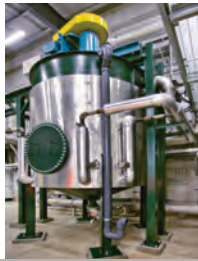
Thermal hydrolysis system from Lystek International
