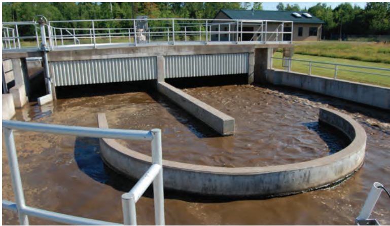
The oxidation ditches at the treatment plant are fed by a blower fitted with a variable-frequency drive.
