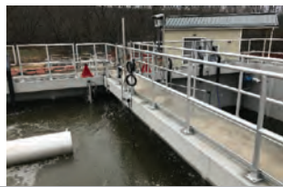
SAM biological wastewater treatment process from Fluidyne
