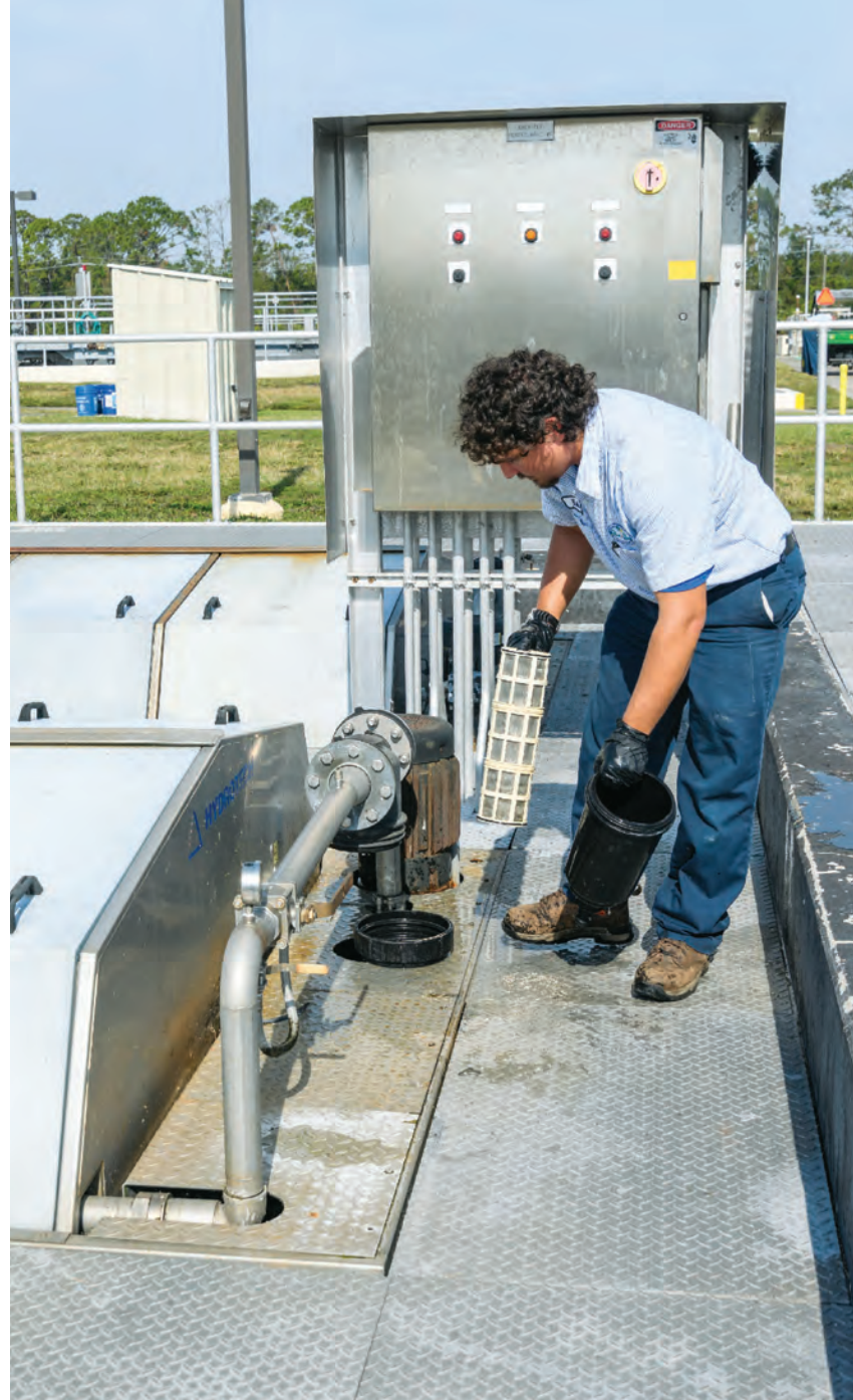
Eric Stodola cleans one of four Hydrotech Discfilters (Kruger), used for tertiary treatment to meet the plant's TSS effluent requirements.
