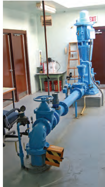
A wellhead pump lifts groundwater to fill the city’s main reservoir.
