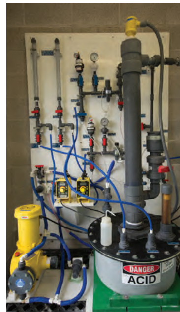
Fluoridation injection pumps (LMI Pumps) at the Church Well fill station.
