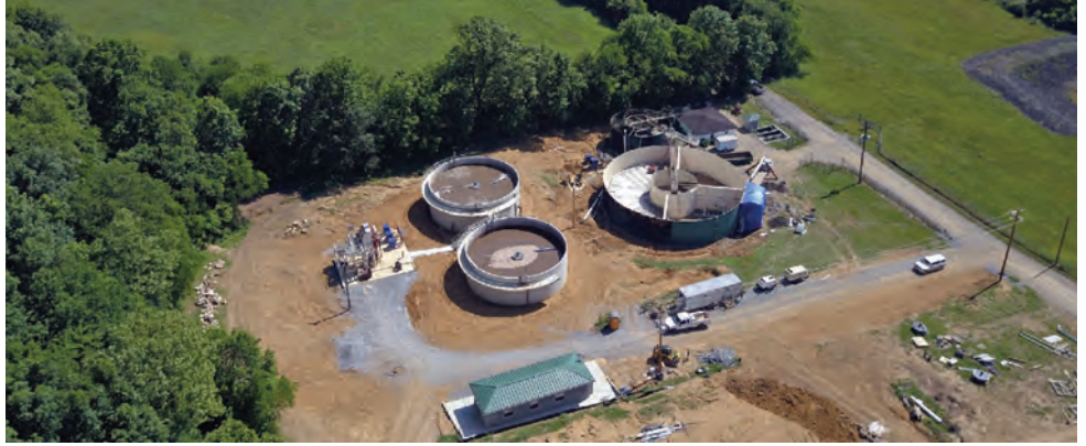
The SBR system (Parkson Corp.) includes the two concrete tanks on the left. The large metal tank (shown while under construction) includes the post-equalization basin and two digesters. The chlorine contact chamber is on the far left.
