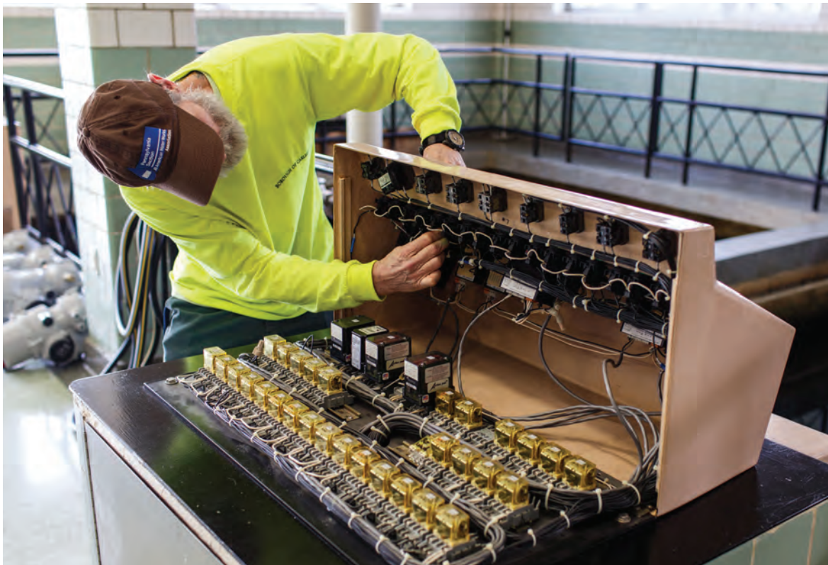
Rick Horn, plant mechanic, works on a control panel (Leopold) from the filter gallery.
