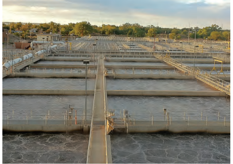
Aeration basins at the Southside plant may undergo an upgrade to a new process with anammox bacteria.
