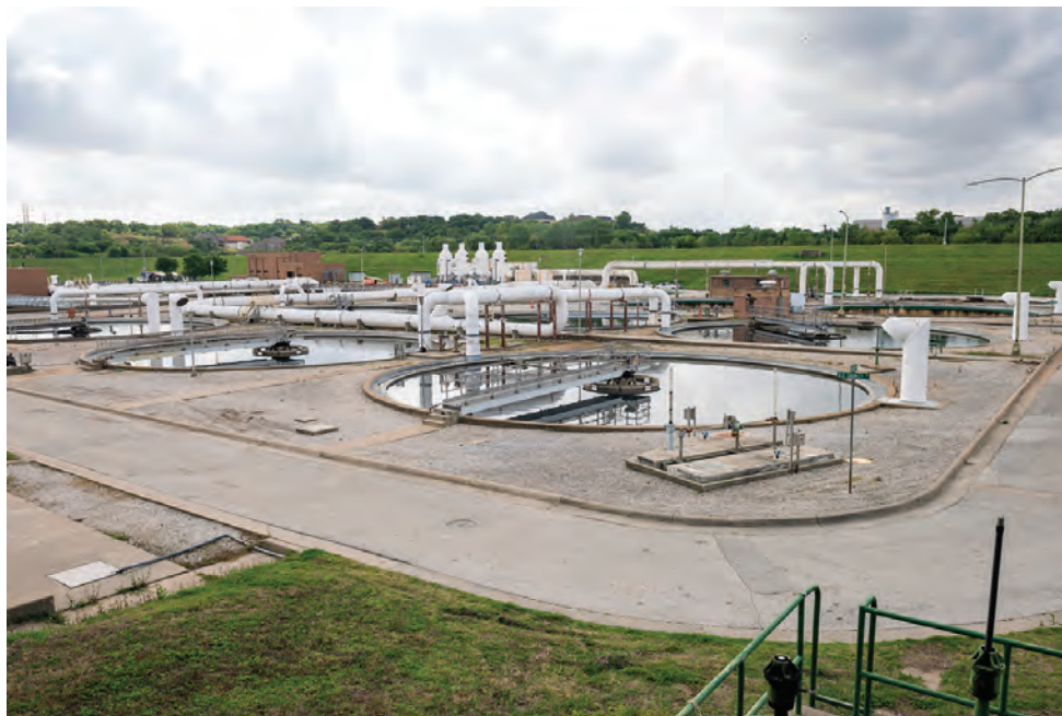
The Village Creek plant treats an average flow of 124 mgd and produces some 28,000 dry tons per year of Class A biosolids for beneficial use.
