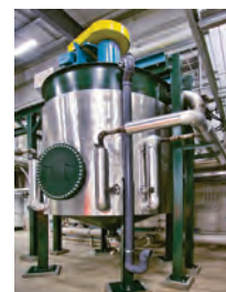
Thermal hydrolysis system from Lystek International
