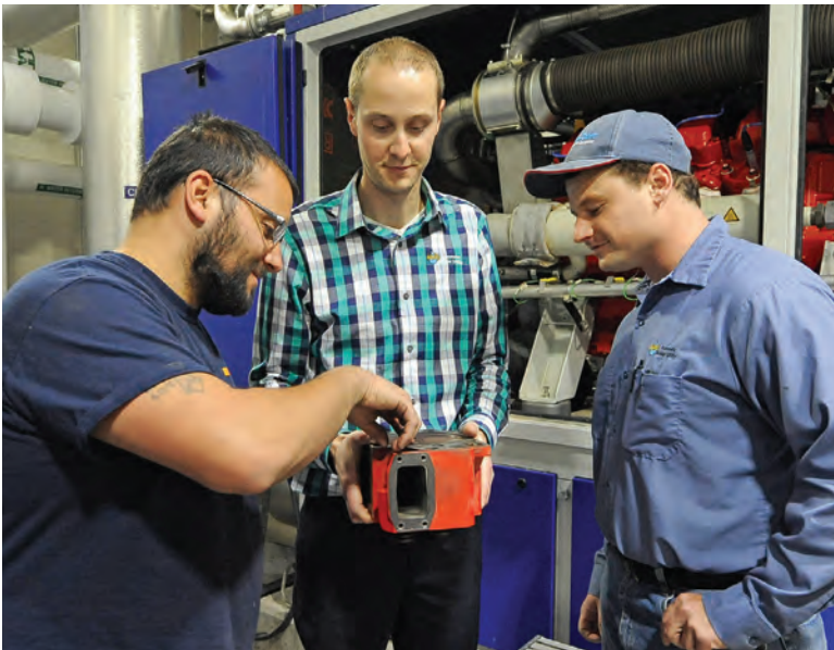
New technology at the plant goes hand-in-hand with basic maintenance. From left, Brian Lequia, Centrisys field technician; Curt Czarnecki and Matt Paul, operator.
