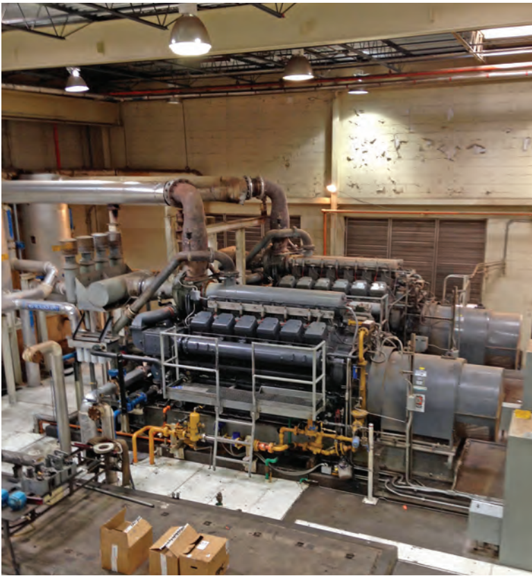
Two 1.1 MW biogas-fueled Cooper Superior engine generators (Eaton) power the plant's South cogeneration system.
