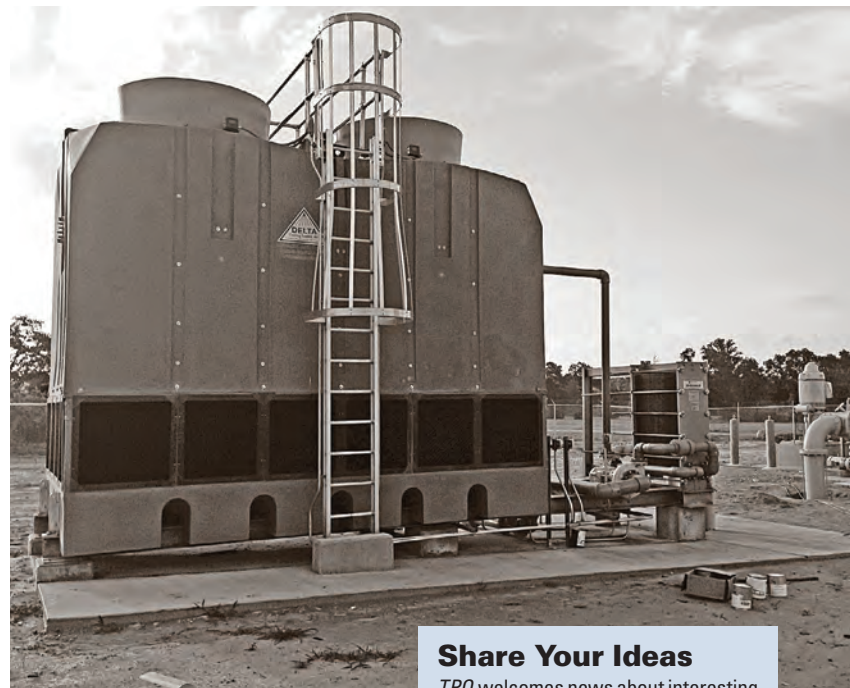
Cooling towers from Delta Cooling reduce the temperature of water from geothermal while also reducing radon and hydrogen sulfide levels.
