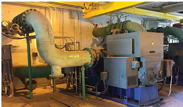
Heat recovered from the plant's cogeneration engine-generators provides hot water for digester heating and reduces natural gas consumption.
