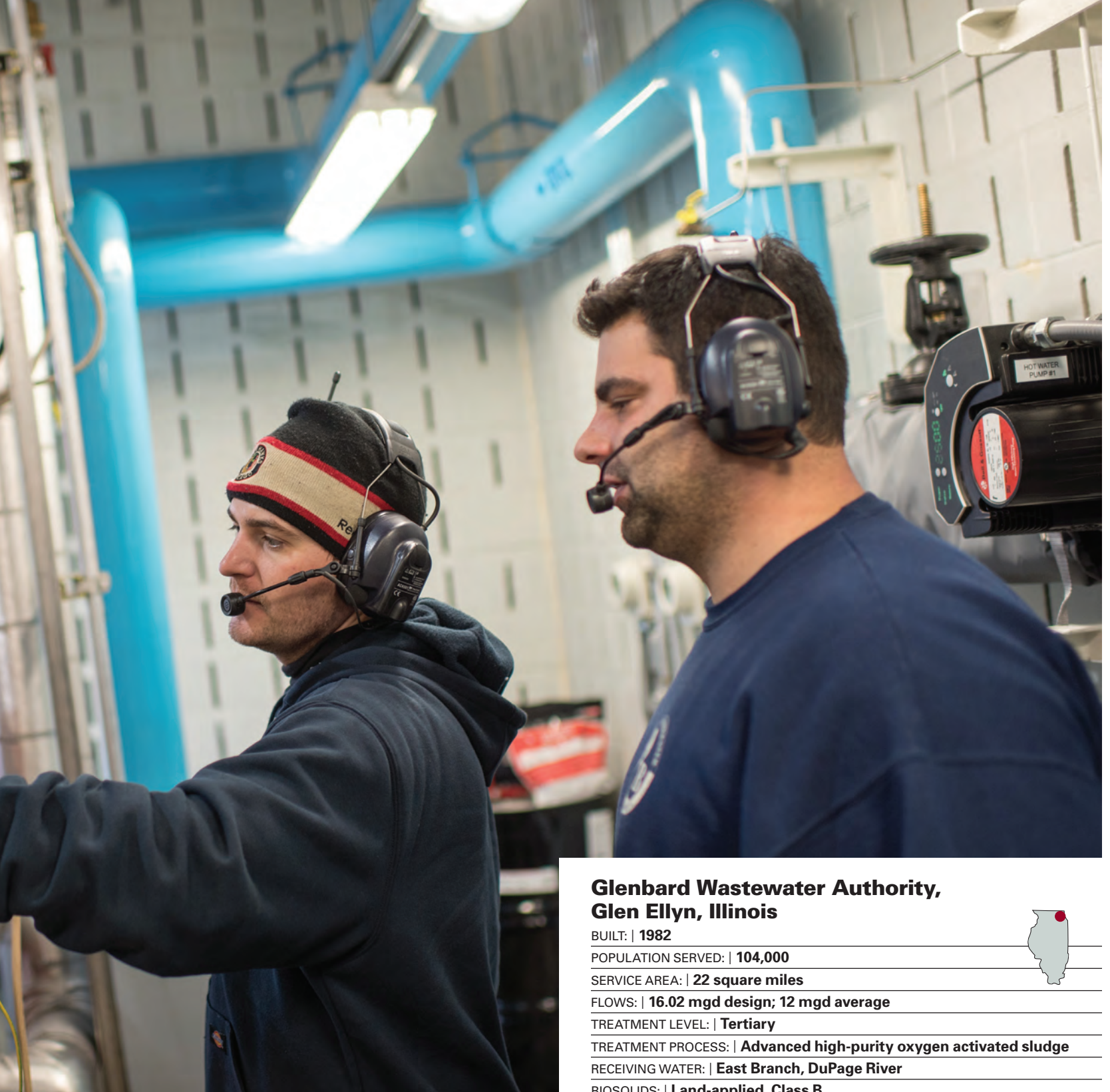
Jon Braga (left) and Austin Cecelia, mechanics, check the combined heat and power engine-generator (Generac) at the Glenbard Wastewater Authority.
