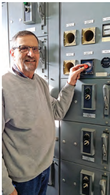
Bob Gabry at the aeration timer control (Eagle Signal).
