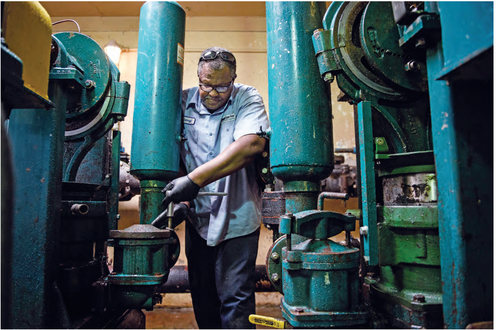
Darryl Tindall, utility maintenance mechanic, services a pump in the primary sludge pump station.
