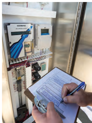
Operators regularly record headworks panel data.
