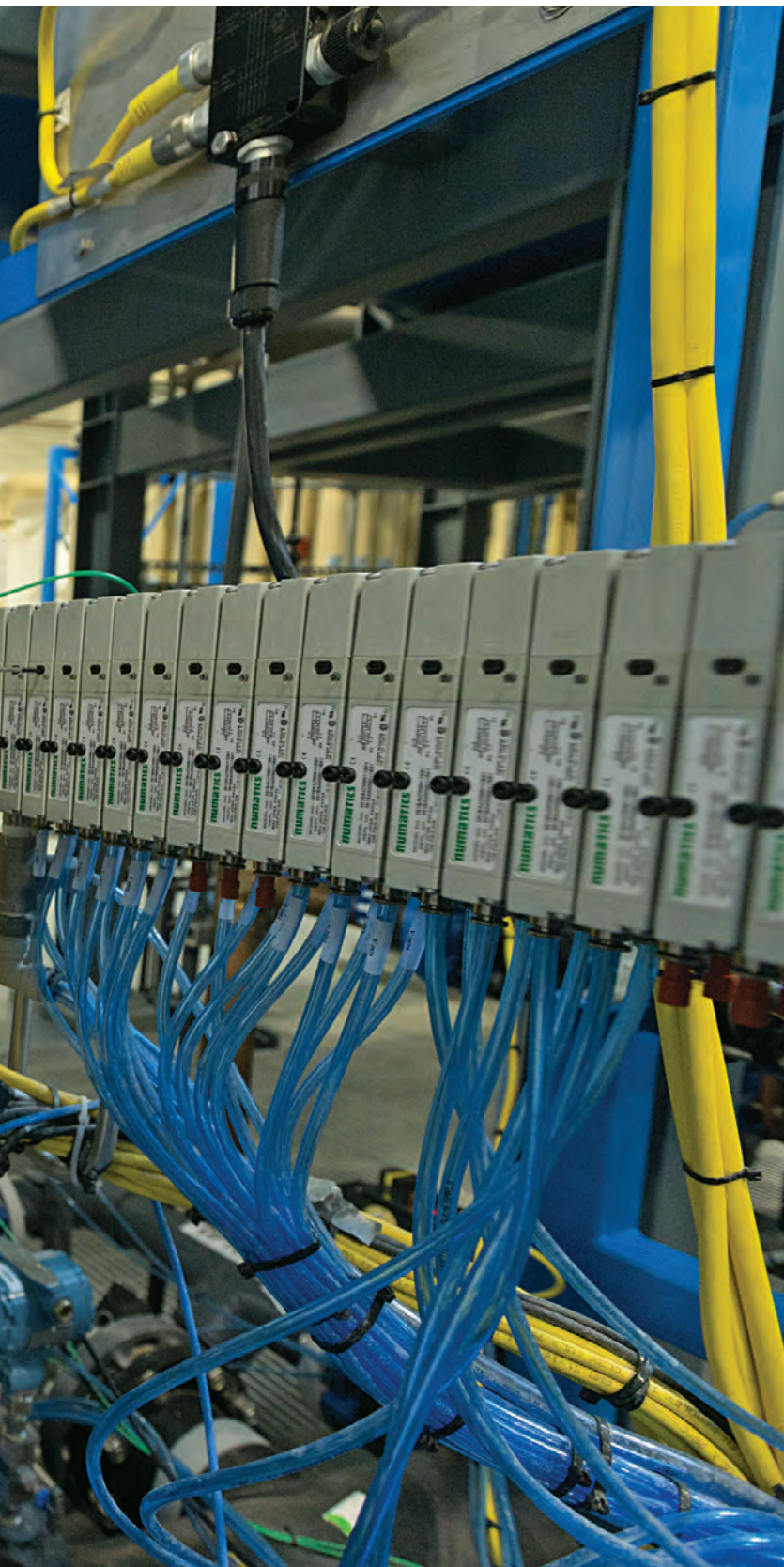
Jordan Hendrix, tradesman at the Ogden City Water Treatment Plant, manually operates an air-actuated valve (ASCO Numatics).
