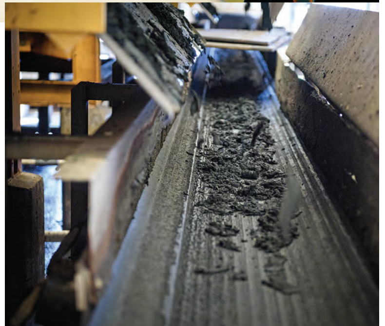
Biosolids cake moves through a belt filter press (Andritz Separation).
