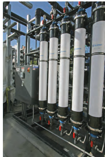
Ultrafiltration is key to the advanced purification process. Recycled water passes through ultrafiltration membrane modules (Scinor).
