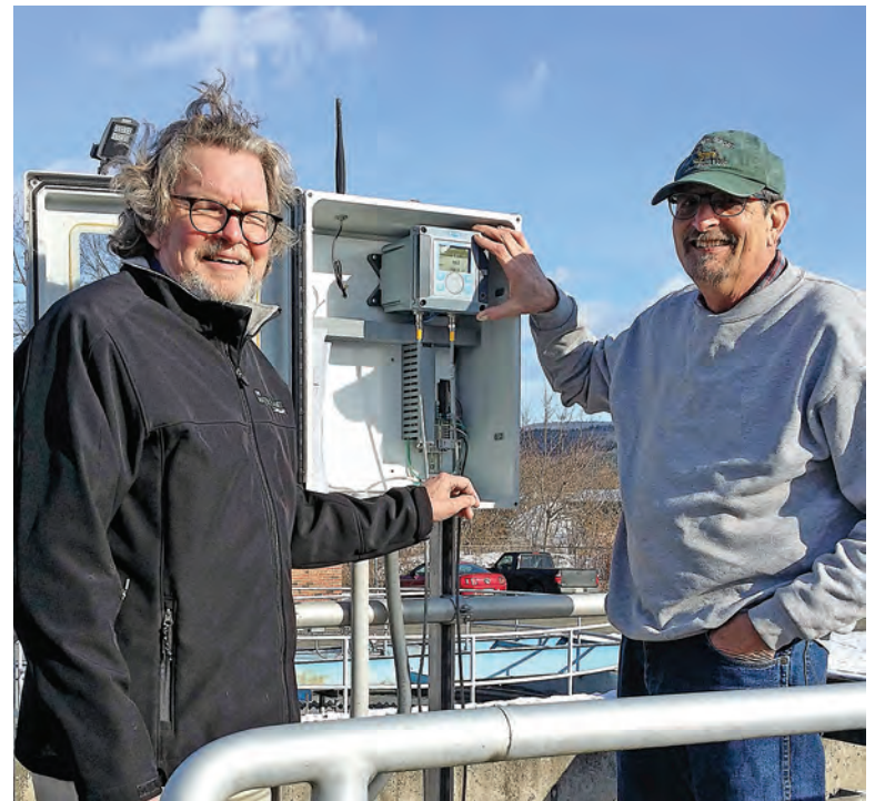
Grant Weaver, left, president of The Water Planet Company, and Bob Gabry, chief operator at the Sunderland Wastewater Treatment Plant, at the MCC panel housing the sc200 controller (Hach).
