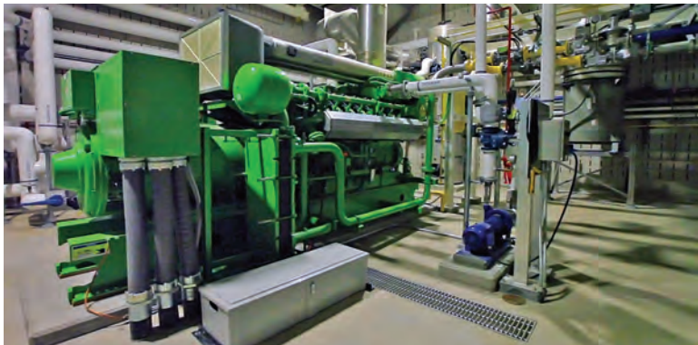
Two 848 kW Jenbacher engines replaced a single 500 kW unit to provide up to 1.7 MW of capacity. A 403 kW SolarCity solar installation provides 450,000 kWh per year.
