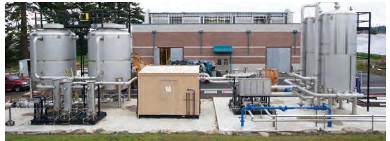
A Unison Solutions gas treatment system is installed outside the cogeneration building.
